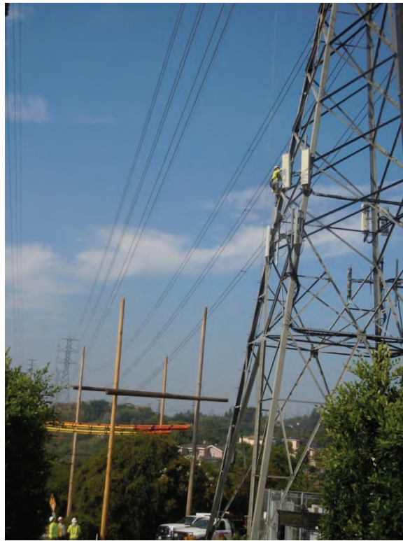
Figure 5: A PAR lineman climbs a tower to remove a traveler after conductor installation, Segment 11A.
