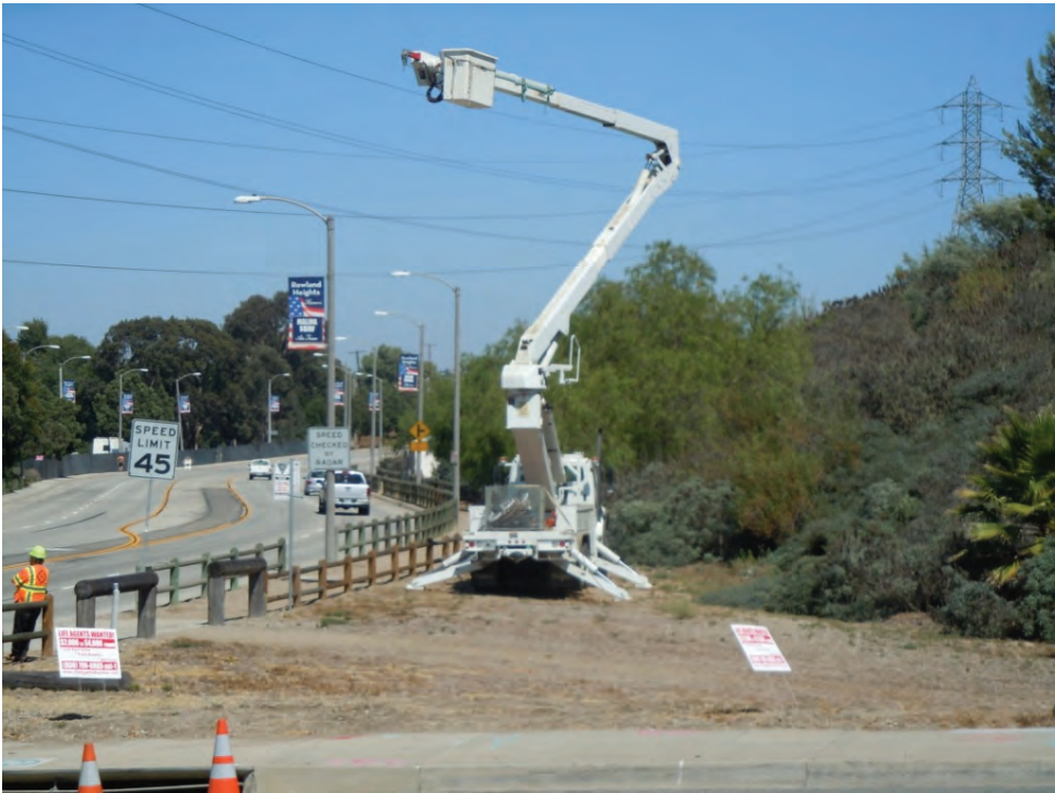
Figure 10: A boom truck parked outside of the area approved as a TEWS request, Segment 8 Phase 4.
