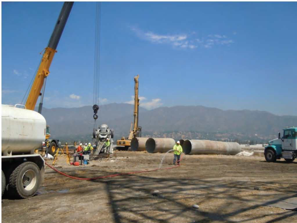
Figure 6: A Tri-State crew pours a foundation while watering for dust control, Segment 7.
