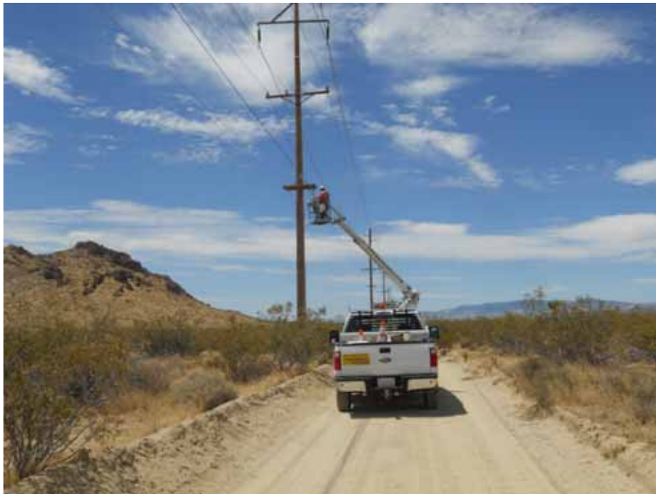
Figure 3: H&M crew adjusting the cable arms on wood poles on Favorito Road, Segment 10 Telecom.
