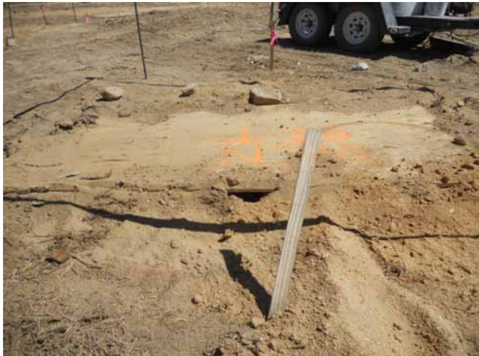
Figure 4: Gap in foundation hole cover at Tower 31, Segment 10.
