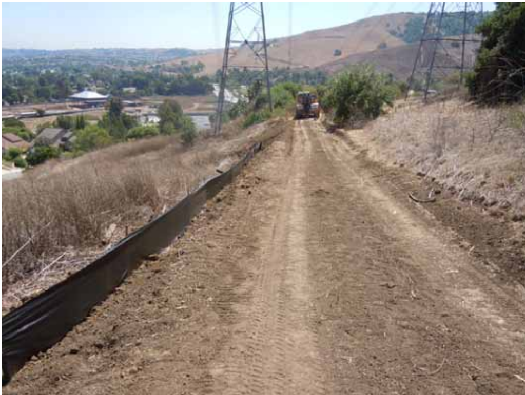
Figure 9: Access road that was unable to support the weight of a crane, Segment 8, Phase 4.
