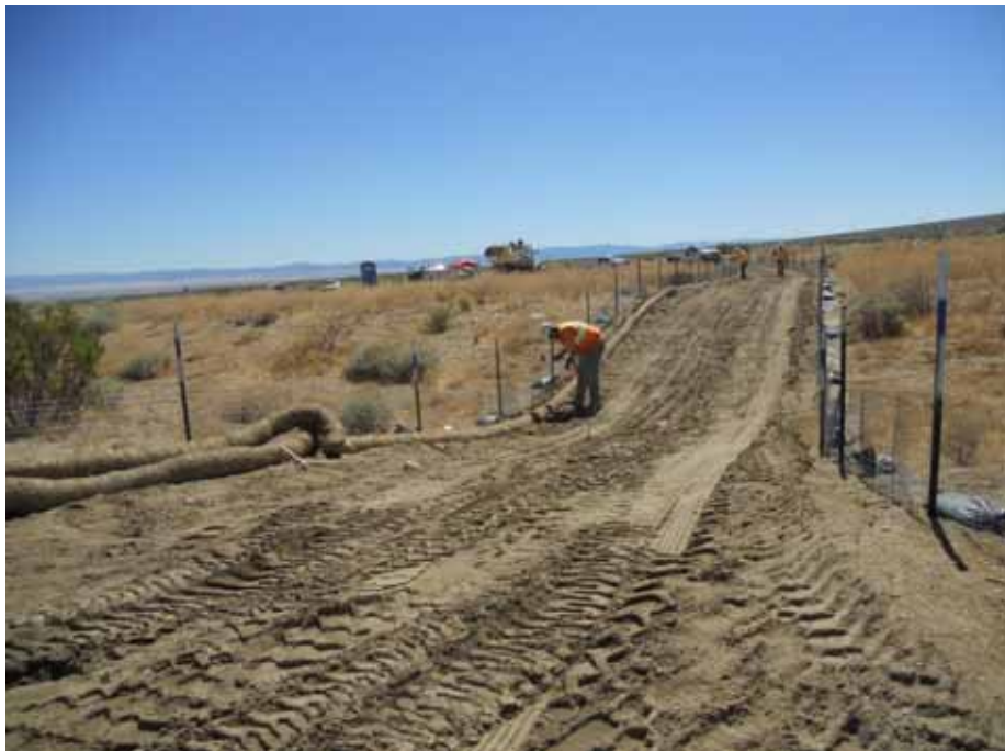
Figure 2: H&H Grading installing fiber rolls along the spur road to Tower 24 on the south side of Tehachapi Willow Springs Road, Segment 10.
