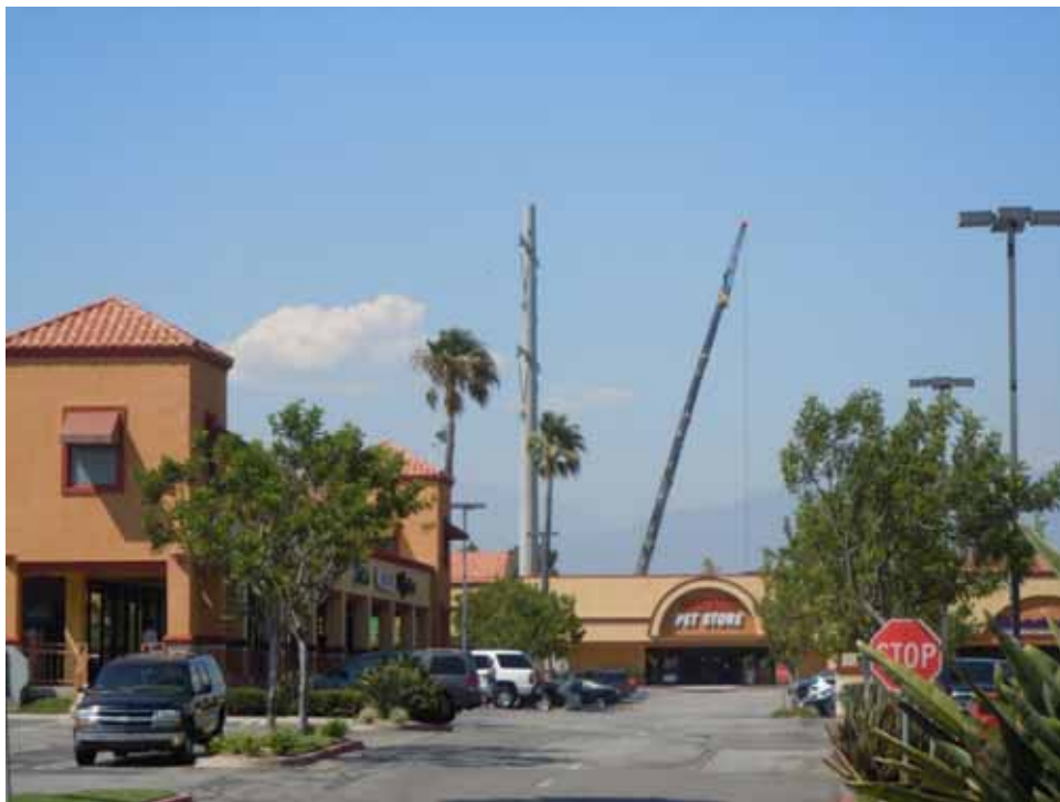
Figure 8: Erection of a TSP as seen from an adjacent mall, Segment 8 Phase 1.
