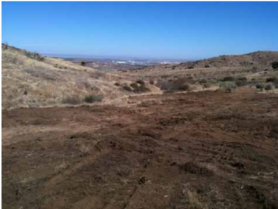
Figure 3: H&H Grading cleared and grubbed the wire set-up site south of Tower 51A, Segment 5.
