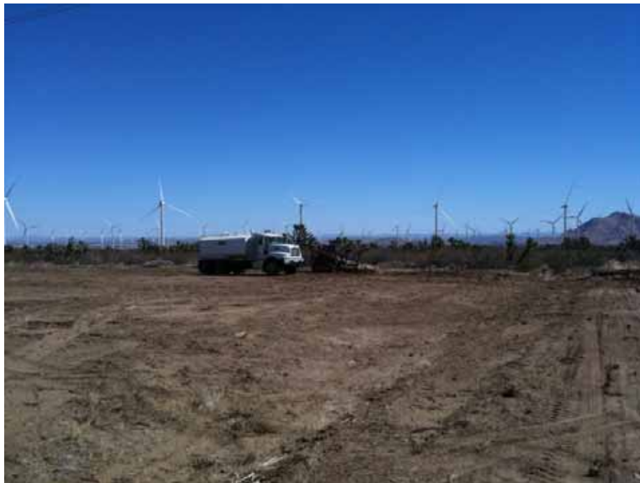
Figure 4: H&H Grading mulched Joshua trees in the wire set-up site at Tower 1, Segment 10
