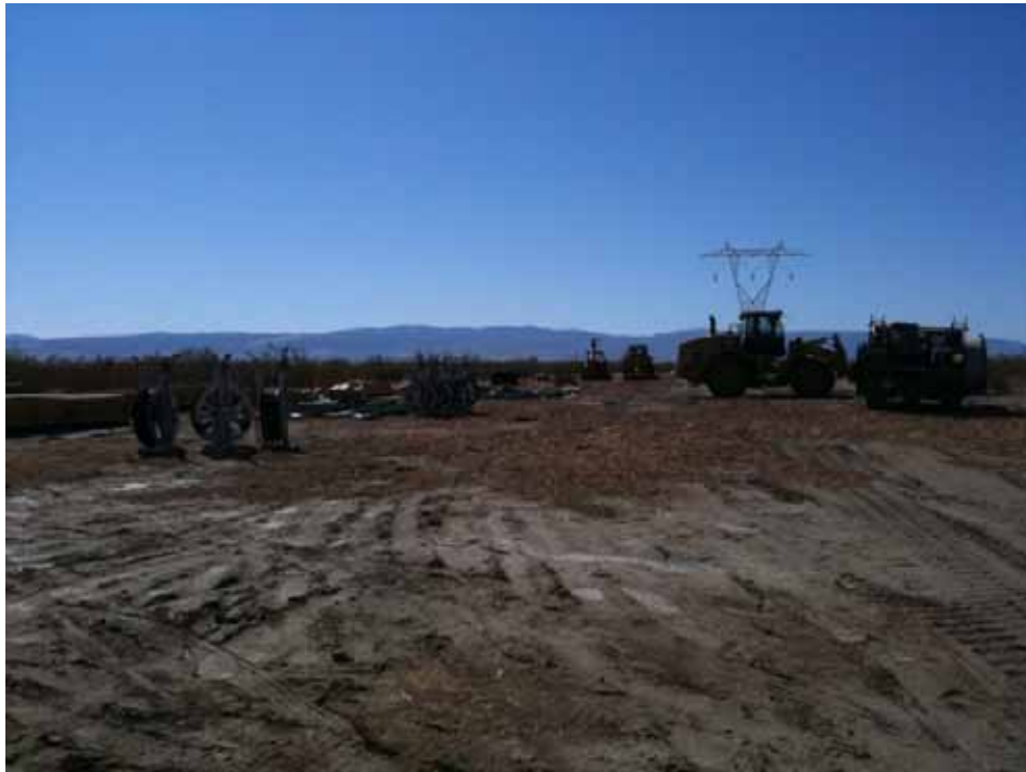
Figure 2: Wire stringing materials being hauled to wire set-up site between Towers 83 and 84, Segment 10 in preparation for wire stringing.
