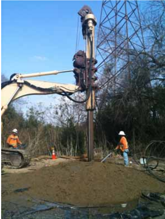
Figure 4: Foundation drilling along Siphon Road in Whittier Narrows with spill pile, Segment 8 66 kV.
