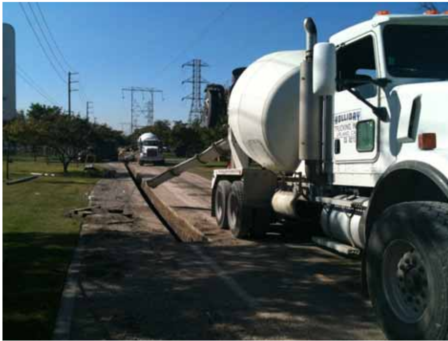
Figure 5: Concrete pour in a distribution trench in Ayala Park, Segment 8 66 kV underground.
