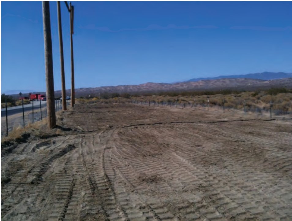
Figure 3: Guard pole site on the north side of Rosamond Boulevard where vegetation was completely removed, Segment 10.
