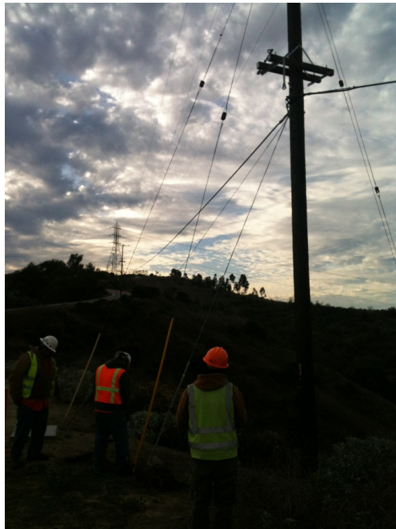
Figure 4: Segment 8 Telecom within Rose Hills.
