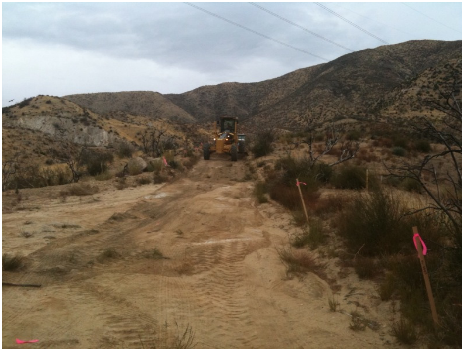
Figure 3: Grading access road that leads to Tower 22 in the Angeles National Forest, Segment 6A.
