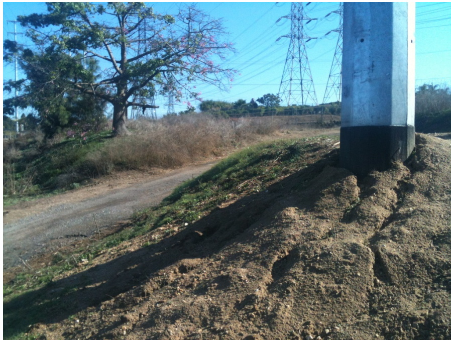
Figure 7: A newly installed 66 kV lightweight steel pole after a rain event, Segment 7.
