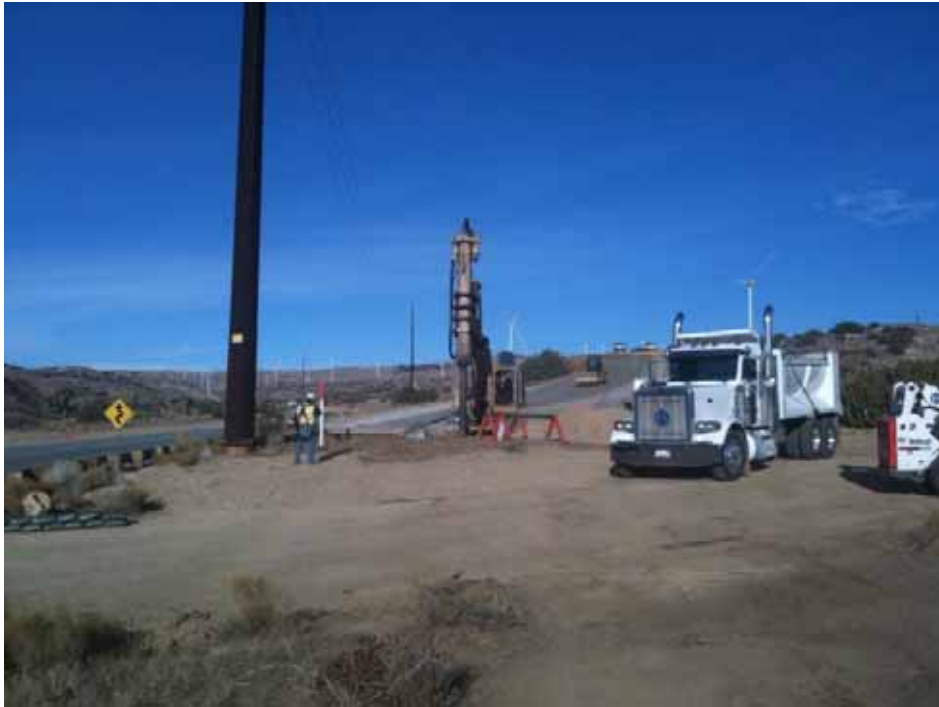
Figure 1: TSP foundation drilling along Oak Creek Road, Wilderness Line, Antelope Transmission Segment.
