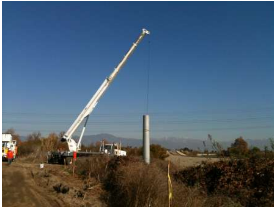
Figure 5: Crews install a light weight steel pole within Whittier Narrows, Segment 8, Phase 4.
