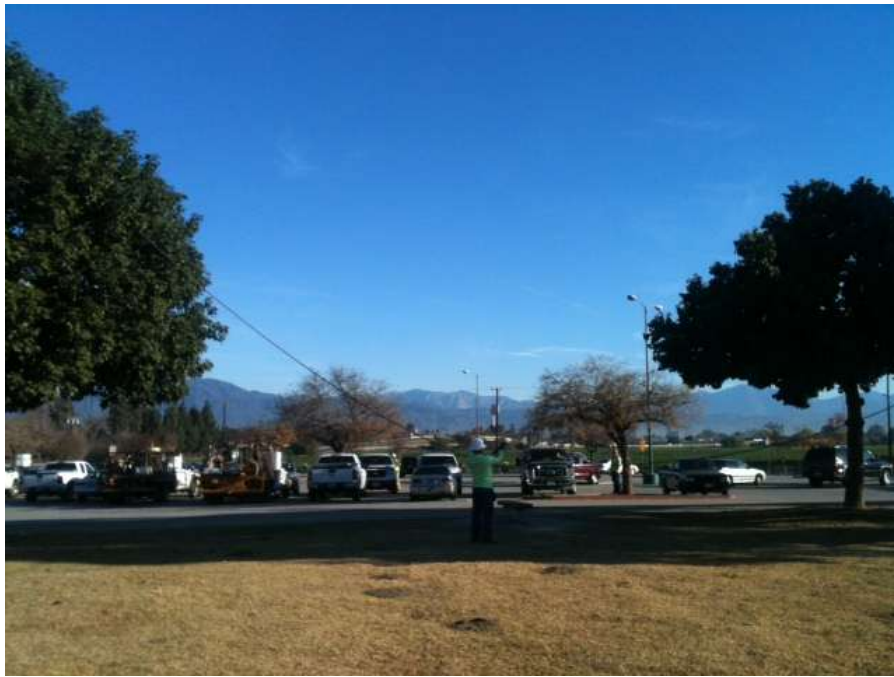
Figure 5: Crews remove conductor from the Rio Hondo–Amador-Jose-Mesa 66 kV line within Whittier Narrows at Legg Lake, Segment 7.
