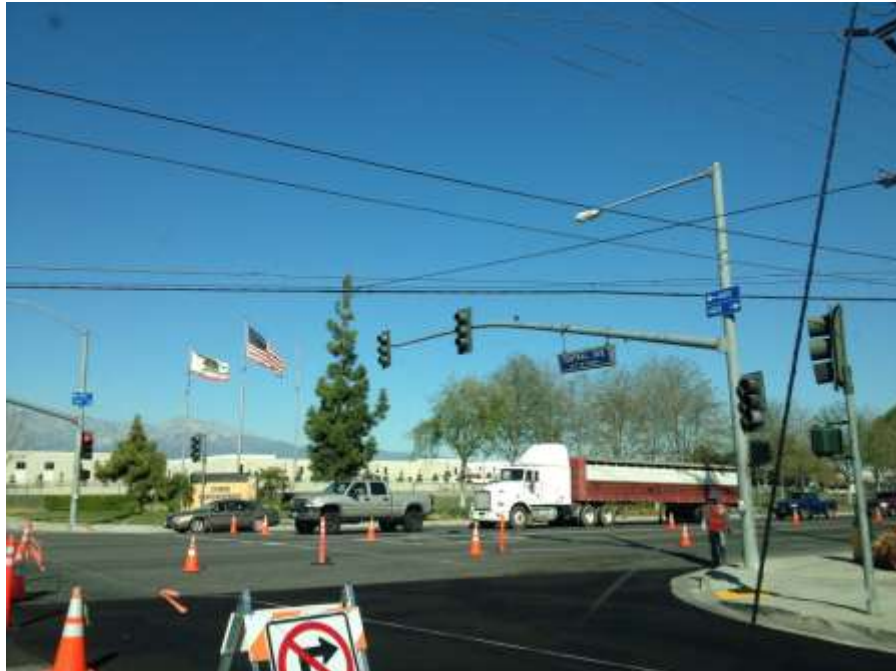
Figure 4: Newly paved road and traffic control at the corner of Central Avenue and Edison Avenue, Chino 66 kV Relocation, Segment 8.
