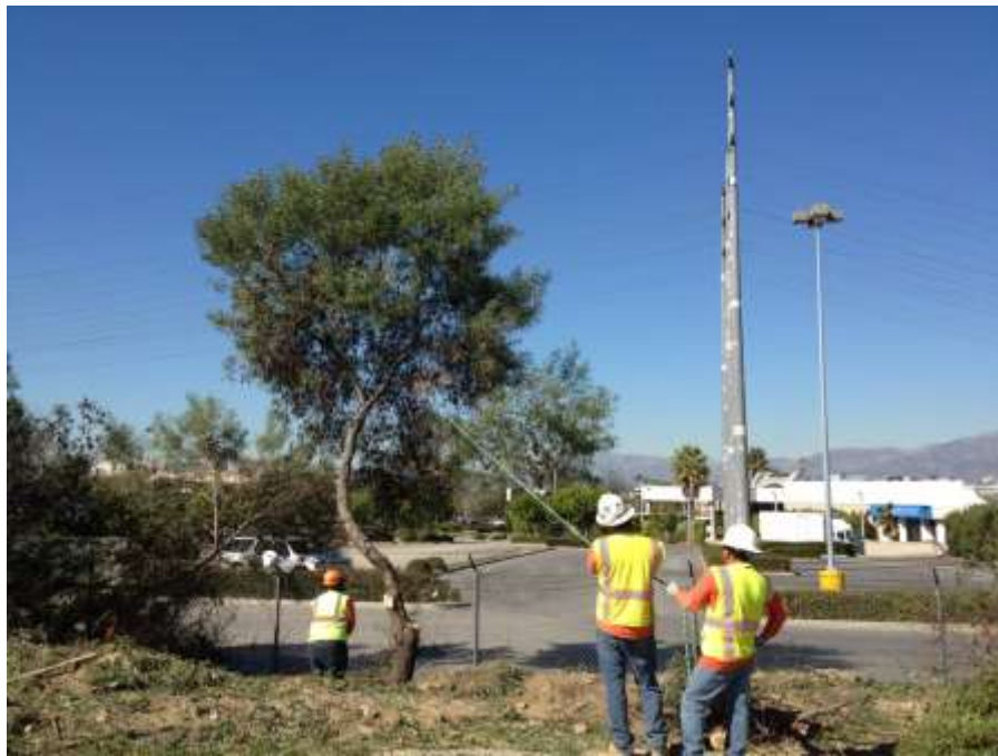
Figure 5: Tree removal during clearing and grubbing at Tower M40-T5 in Montebello Hills, Segment 7.
