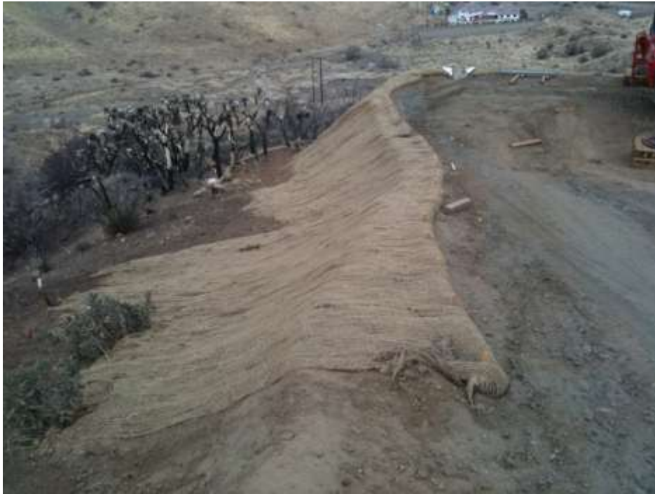
Figure 1: H&H Grading steel crew installed jute netting on slope at Tower 25, Segment 5.
