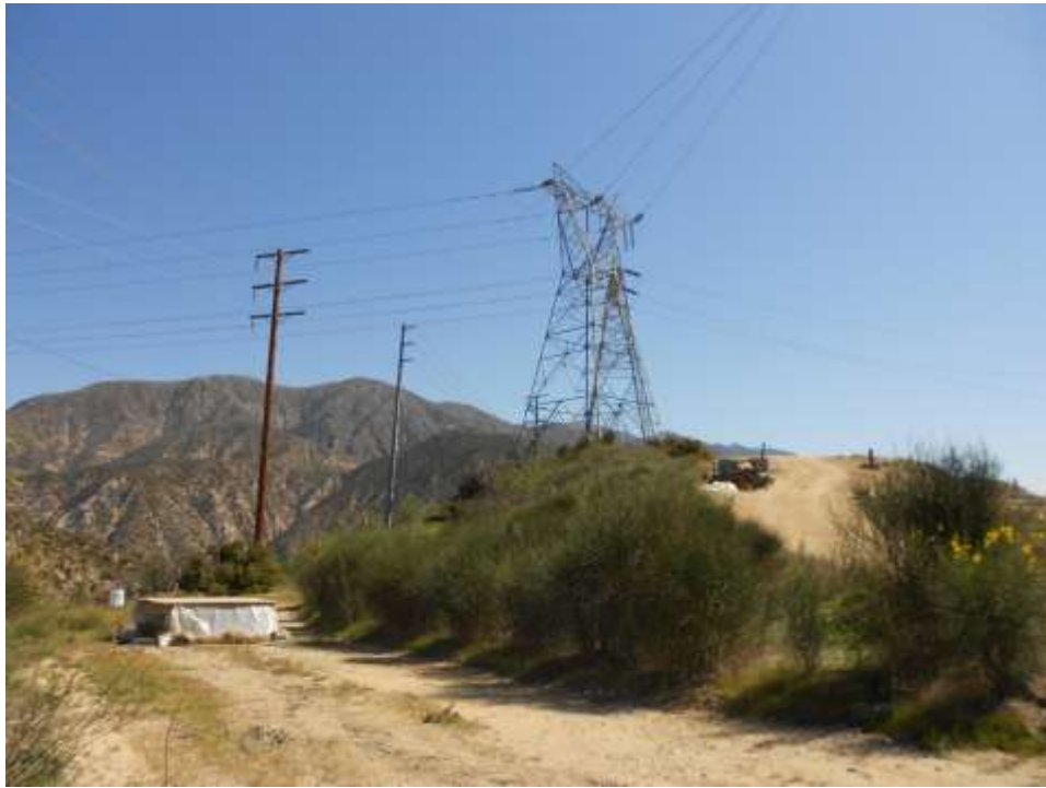
Figure 3: Newly established concrete washout and new structure foundation at Gould substation, Segment 11D.
