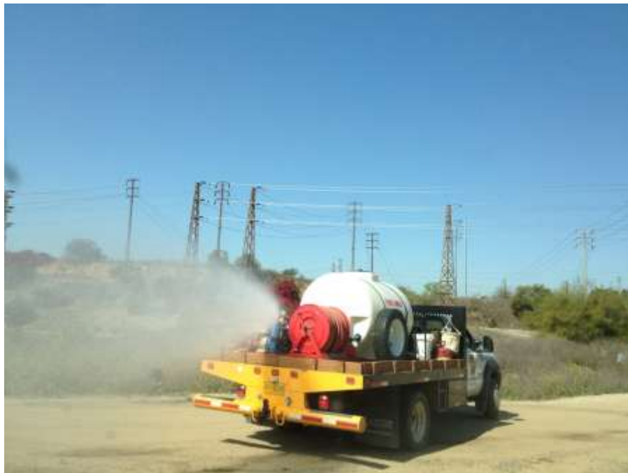
Figure 6: Dust control suppression during stringing preparation between towers M42-T5 and M42-T6, Segment 7.
