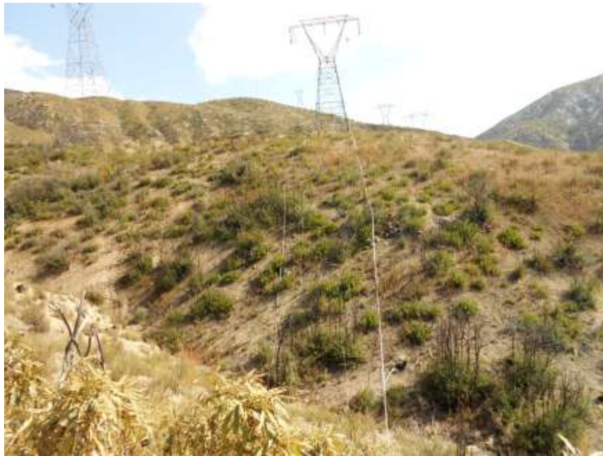
Figure 4: Conductor placed on ground during wire removal between Towers 62 and 63, Segment 6B.
