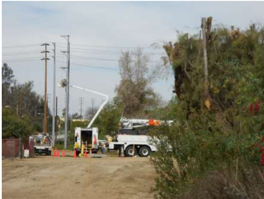
Figure 5: A 66 kV crew installs hardware on a pole, with an ESA for a bushtit nest shown in the foreground.
