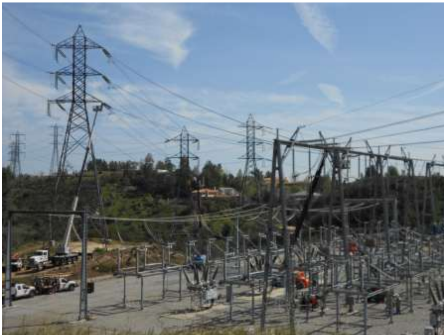
Figure 4: Crews remove wire adjacent to a raven nest, Segment 11D.
