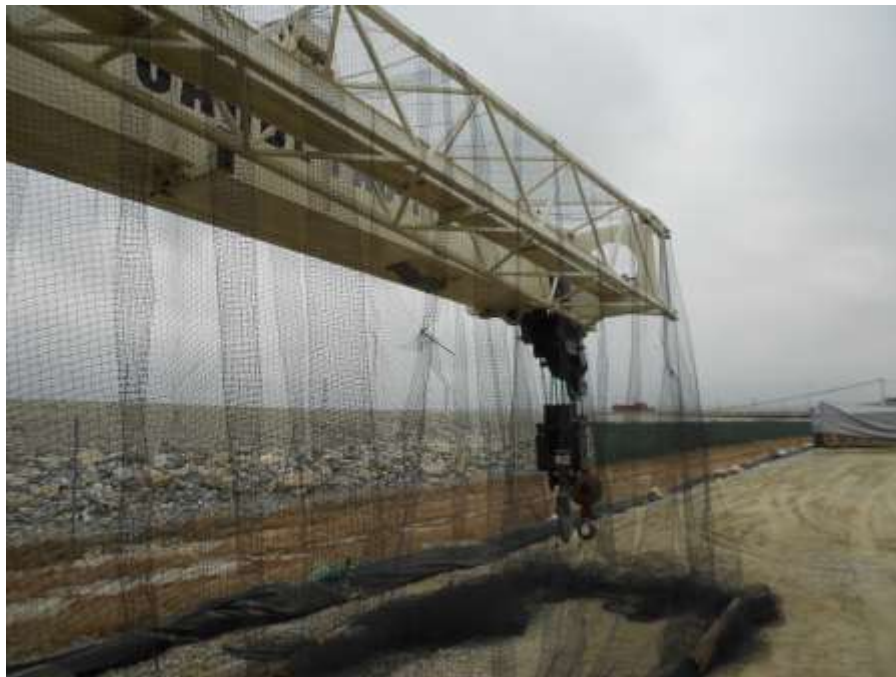
Figure 8: A repaired hole in bird deterrent netting, Segment 7.
