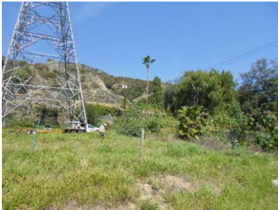
Figure 7: A crew member mows the tower site in preparation for hydroseeding, Segment 7.
