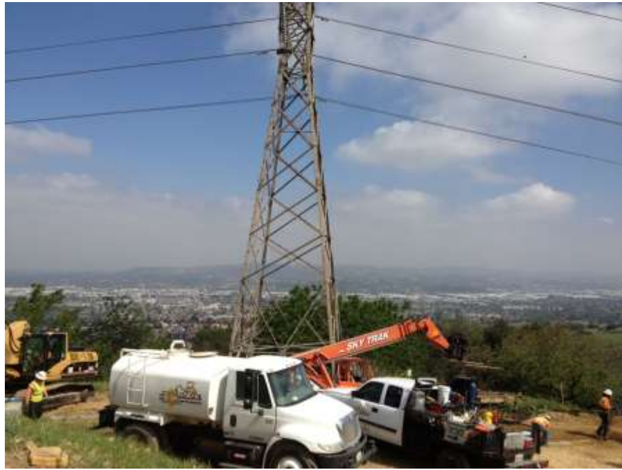
Figure 5: A DCX crew prepares a site for a foundation drilling with a common raven nest in the background, Segment 8 Phase 4.
