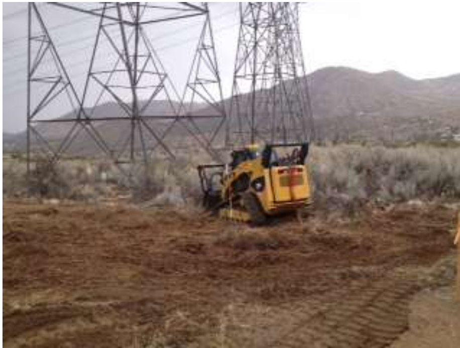
Figure 3: Vegetation removal within an approved nest buffer reduction at Construct 7, Segment 6A.
