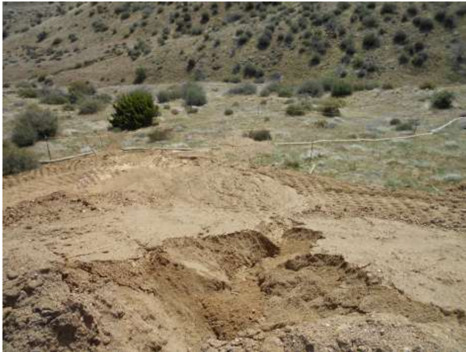
Figure 2: Erosion at Tower 86A, Segment 5.
