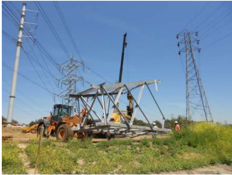
Figure 7: A crew moves a tower section within a CAGN buffer, Segment 8, Phase 4.
