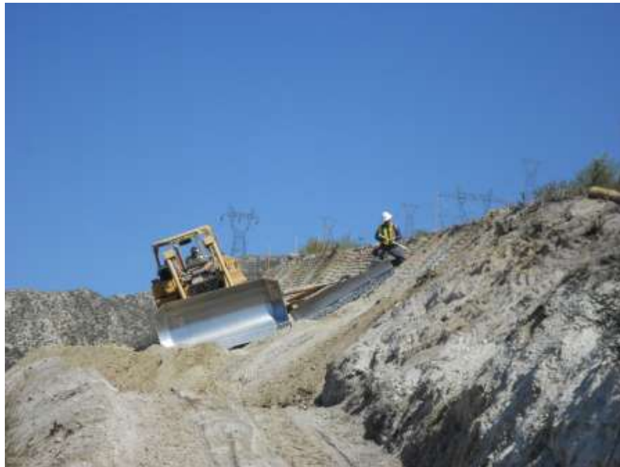
Figure 4: A crew grading a road and wall on Loop Road F, Segment 6B.
