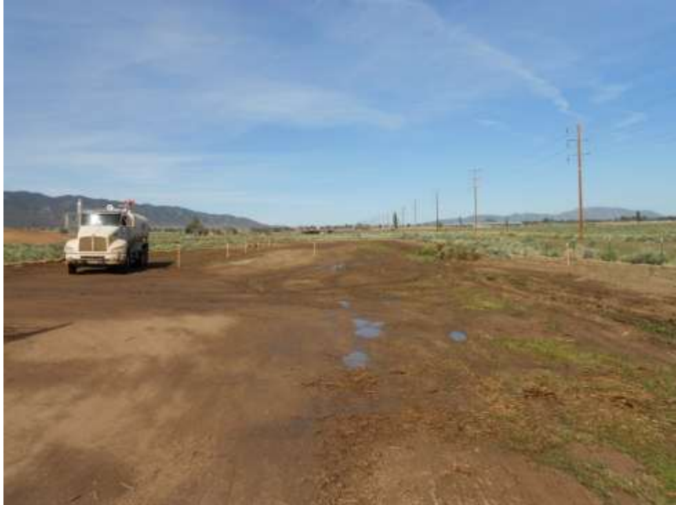
Figure 2: Grubbing activity for the new permanent access road into the Highwind Substation, Segment 3B.
