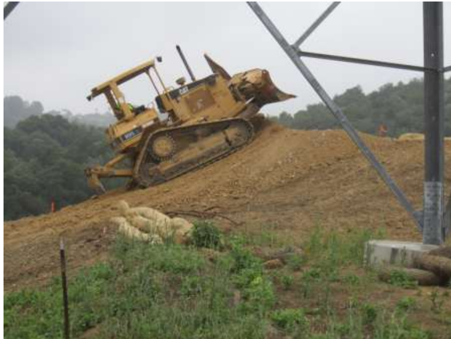
Figure 6: A bulldozer track walks a site above a newly constructed crane pad, Segment 8, Phase 4.
