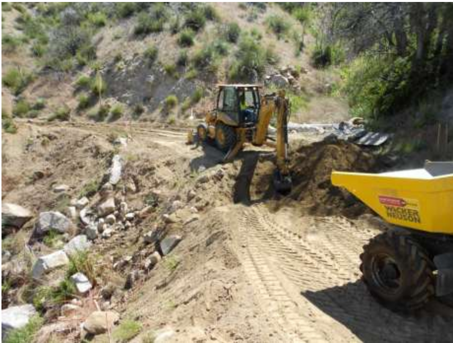
Figure 3: Grading for a gabion wall installation near Structure 64 on Loop Road H, Segment 6B.
