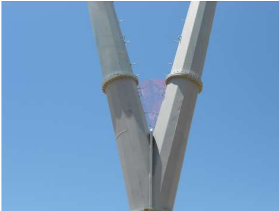
Figure 2: Orange safety fencing installed in the “V” portion of the tubular steel pole (TSP) for bird deterrent netting, Segment 3B.
