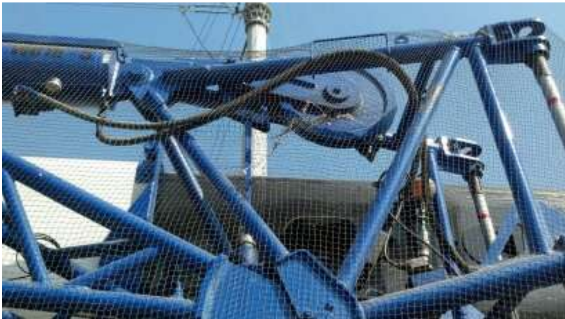
Figure 4: Bird netting over equipment was inspected and holes repaired at the 605 Yard.
