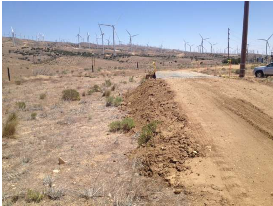
Figure 3: Spoil ramp falling outside the existing road prism at the temporary bridge north of Construct 41, Segment 3B.
