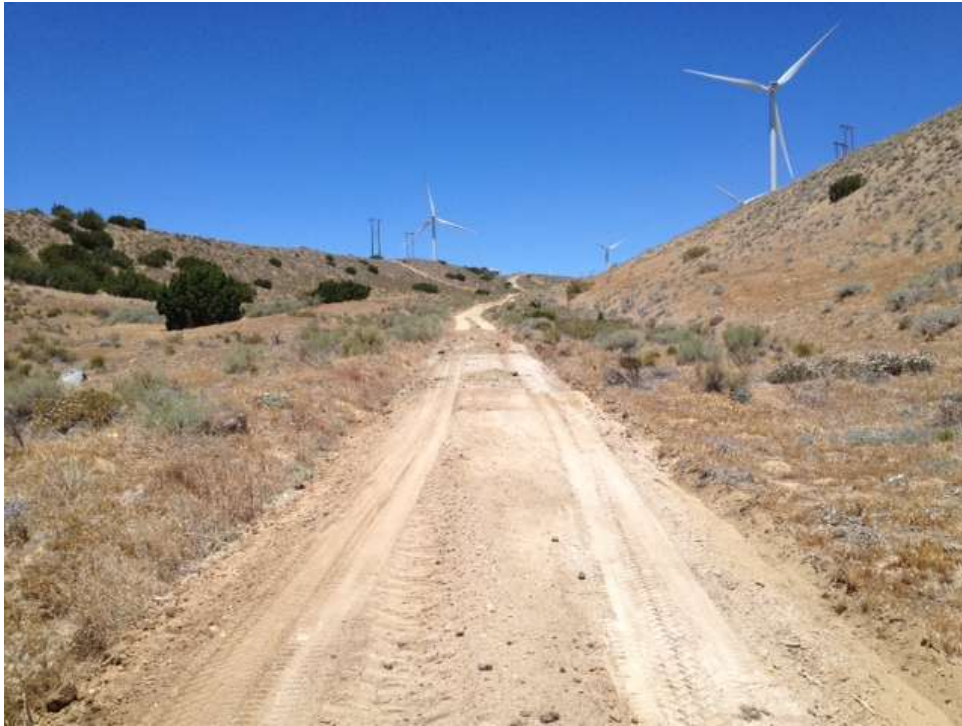
Figure 1: Soil being placed on the access road to Construct 49 for dirt ramp cover over pipeline, Segment 3B.
