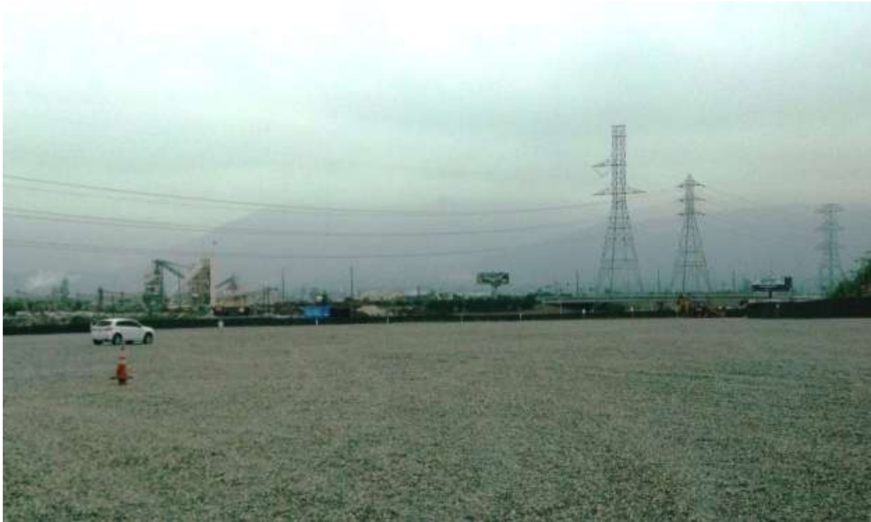
Figure 4: A backhoe (right) moves rock out of a least Bell's vireo buffer while a Biological Monitor (vehicle on left) observes.
