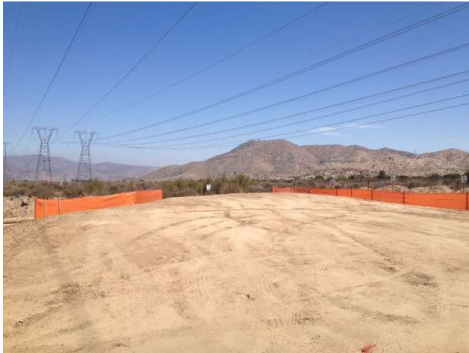
Figure 3: Silt fence installation along salvaged topsoil piles at the WSS at Construct 16, Segment 6A.
