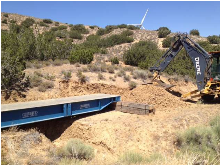
Figure 2: Grading hillside to safely install a Quickbridge over a jurisdictional drainage north of Construct 46, Segment 3B.
