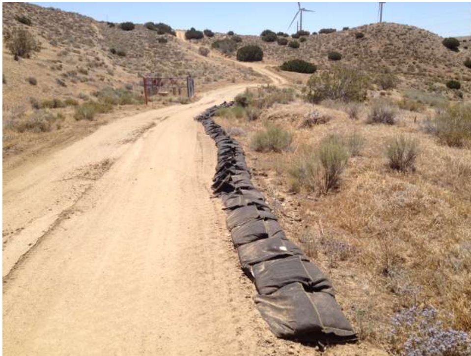
Figure 2: Gravel bags installed along access road to protect a jurisdictional drainage, near Construct 49 on Segment 3B.
