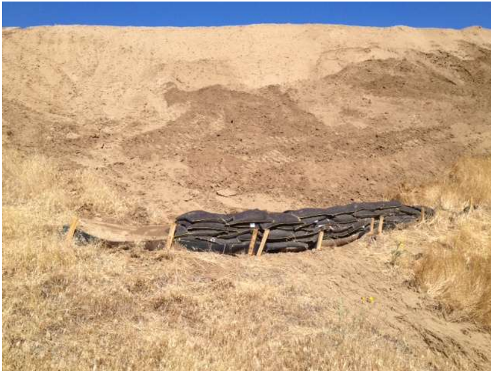
Figure 3: BMP's needing repair from grading and watering activity at Construct 28, Segment 3B.
