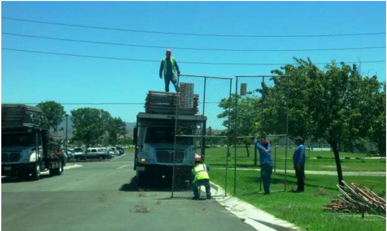
Figure 6: Fence removal in Ayala Park prior to 4 th of July events at the request of the City of Chino.
