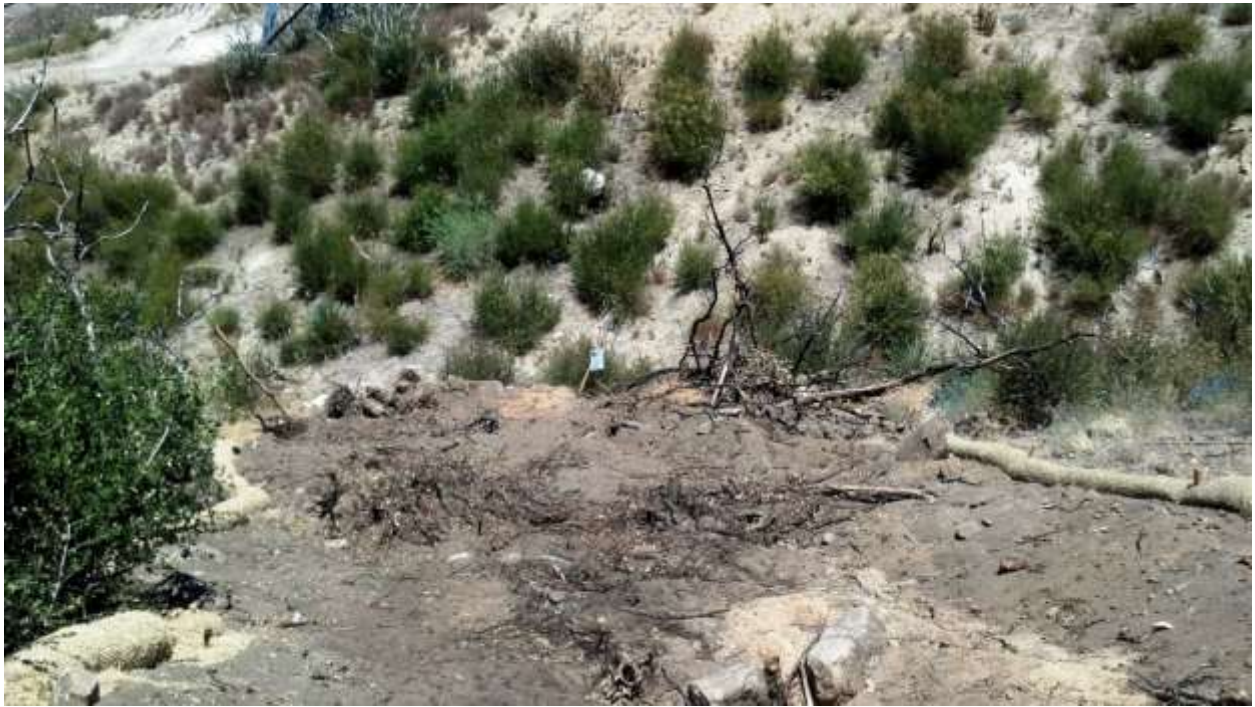
Figure 5: Crews mistakenly graded a cat trail (intended for overland travel only) near Construct 29, Segment 6A.
