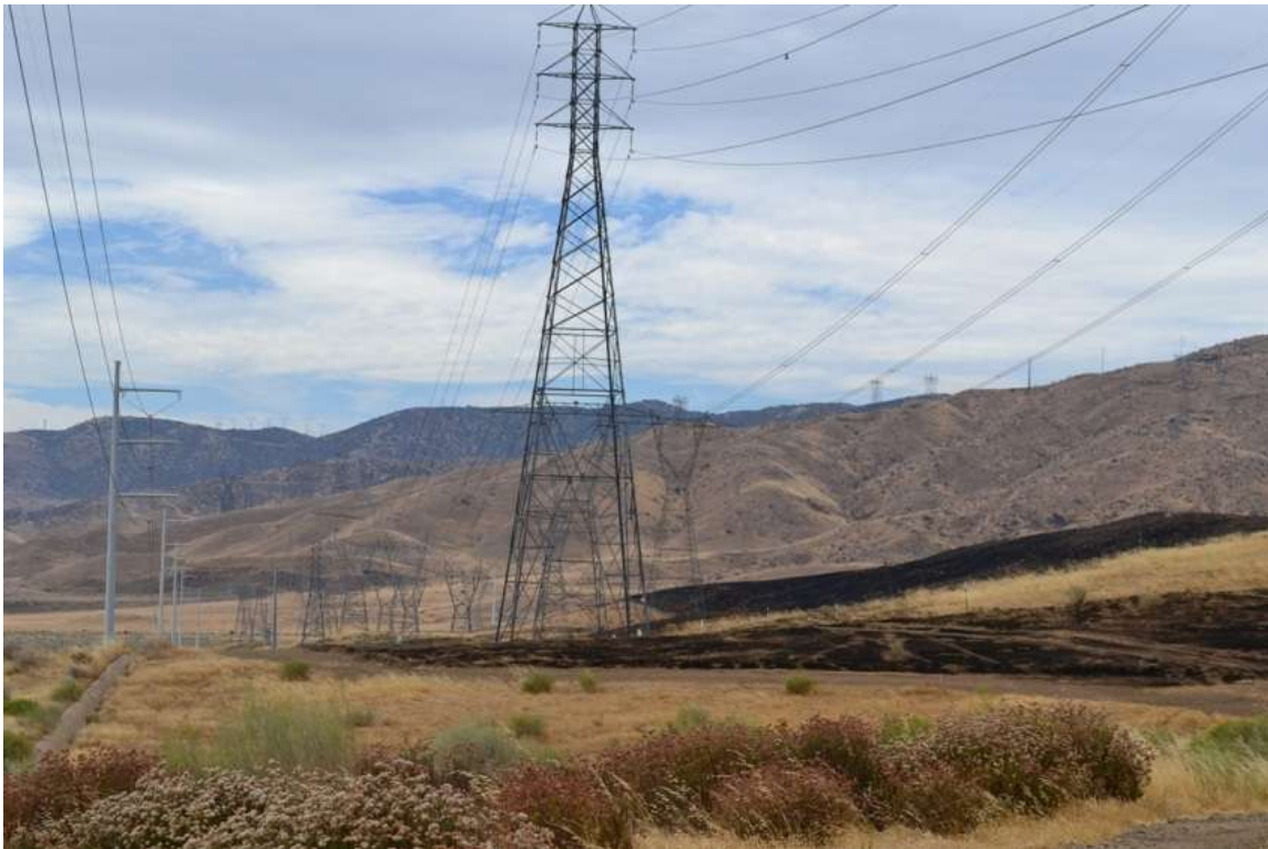
Figure 2: Fire impacted areas of Segment 5 near Tower 37.
