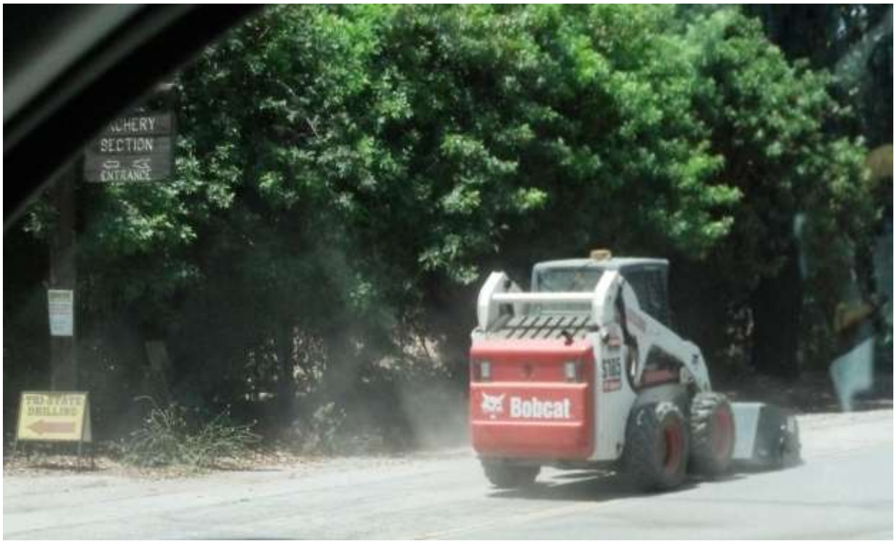
Figure 9: Crews used a street sweeper attachment to remove track-out near Tower 40/1, Segment 7.
