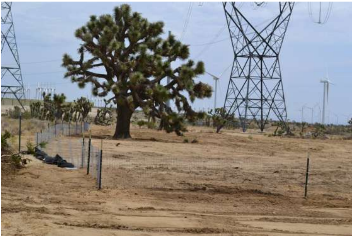
Figure 2: Installation of tortoise fencing surrounding work areas south of Windhub Substation, Segment 10.
