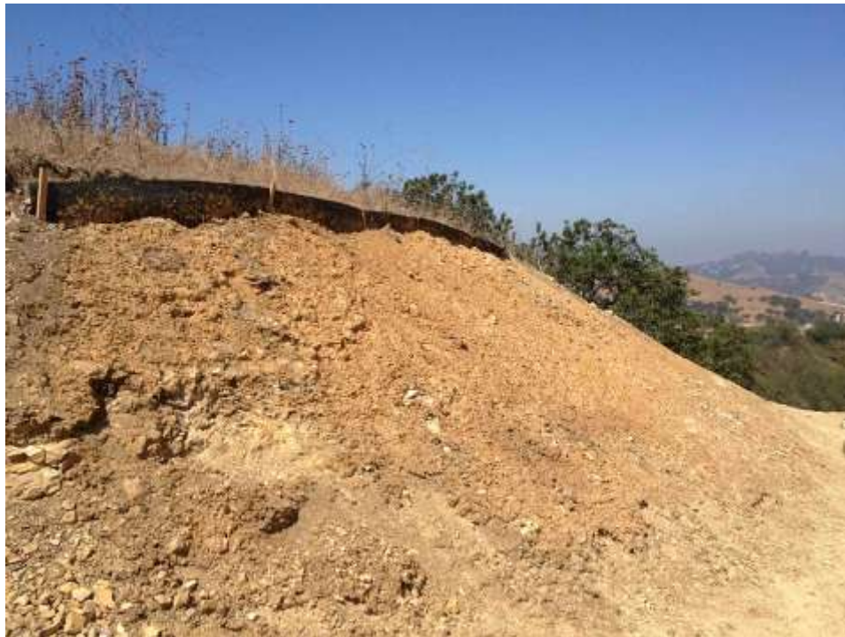
Figure 6: Soil tackifier sprayed on an access road for erosion control, Segment 8, Phase 4.
