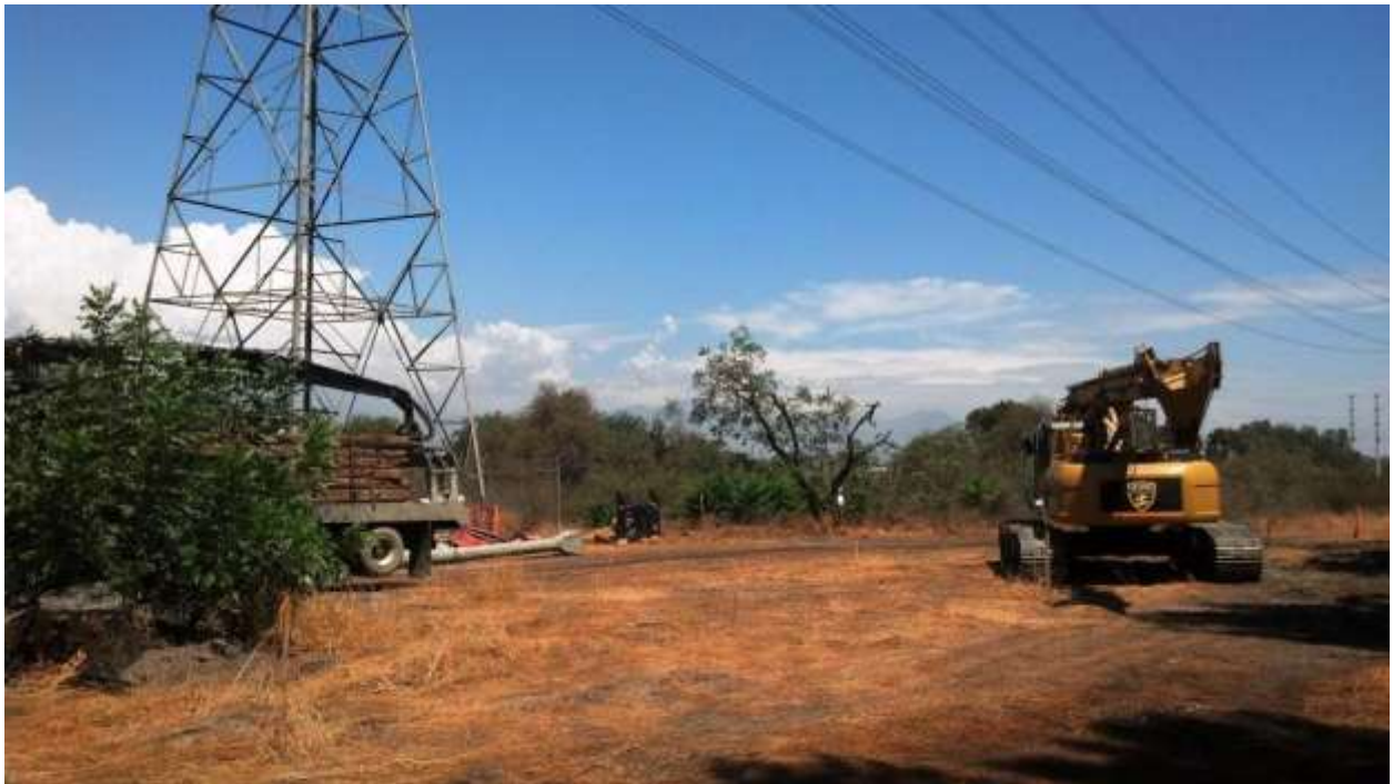
Figure 11: Tri-State drilling crews setting up adjacent to least Bell's vireo habitat at Construct M42-T4 on Segment 8, Phase 4.
