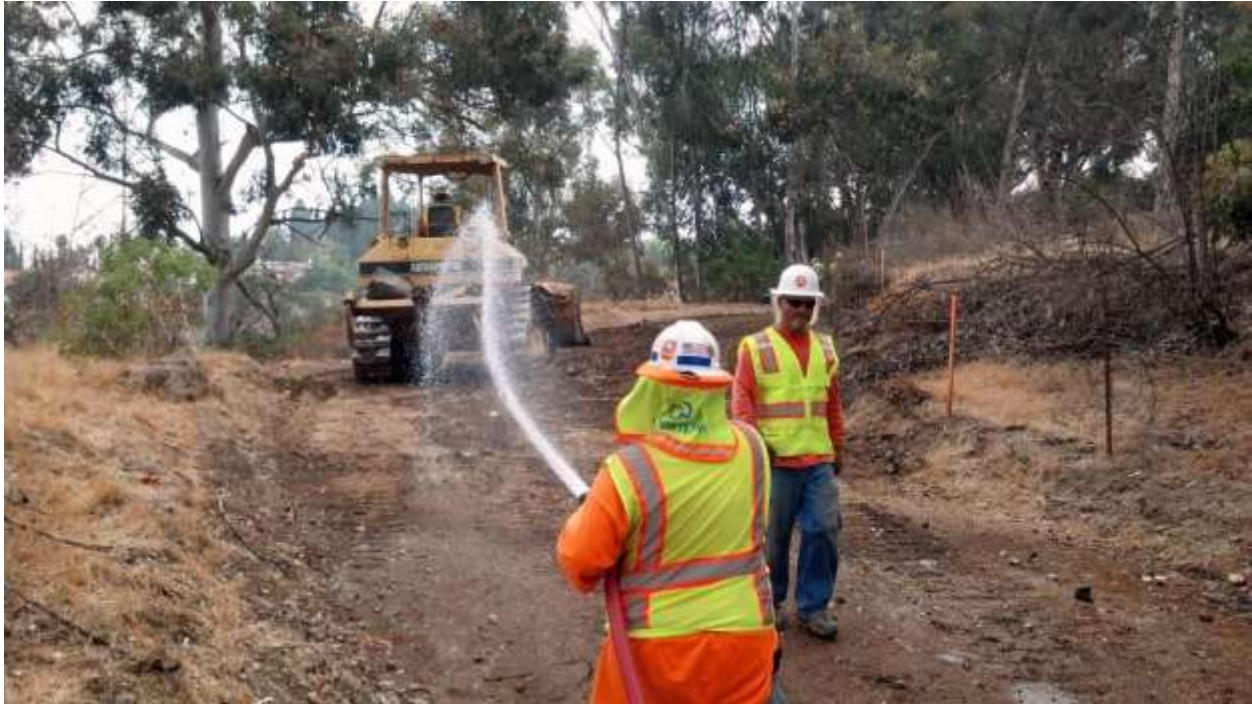
Figure 8: Dust control by DCX in Puente Hills during curve widening on Segment 8, Phase 4.
