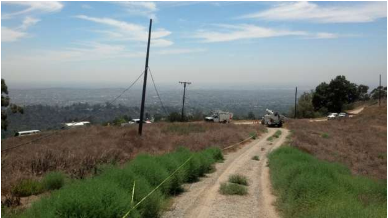
Figure 13: Power lines downed, looking south from communications station.
