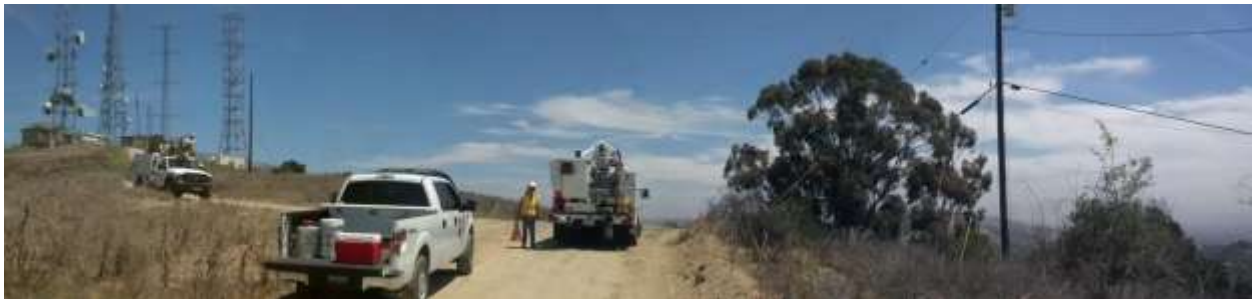
Figure 12: Panorama of drill rig accident site where wires fell in Puente Hills.
