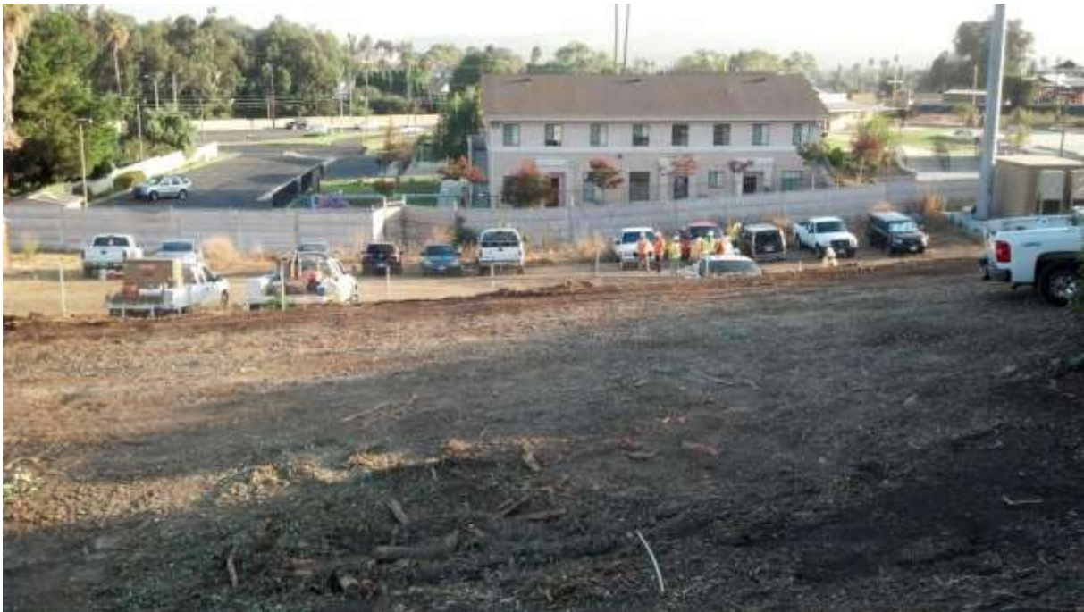
Figure 6: The Fullerton yard was visible from the road once vegetation was removed. Per the project guidelines for visual impacts, a screen was installed the following week.
