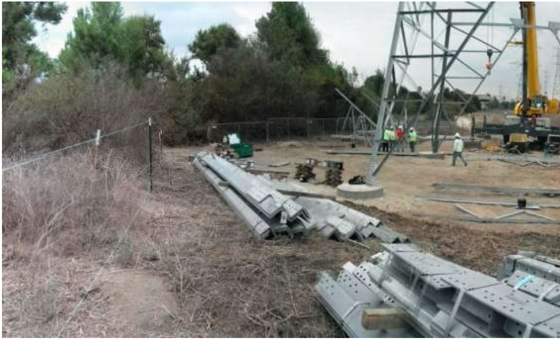
Figure 9: Tower assembly and environmental sensitive areas (ESAs) roped off at M38-T4, Segment 7.
