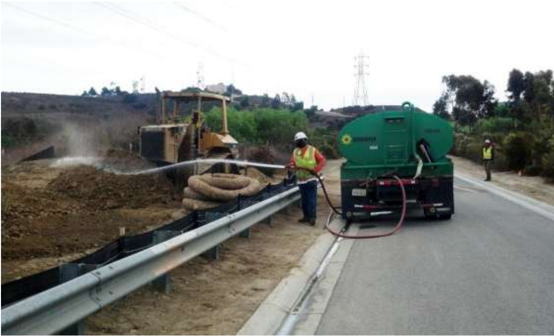
Figure 9: Vegetation clearing and tower pad grading with dust control while Paleontological Monitor (right) looks on at M44-T1, Segment 8, Phase 4
