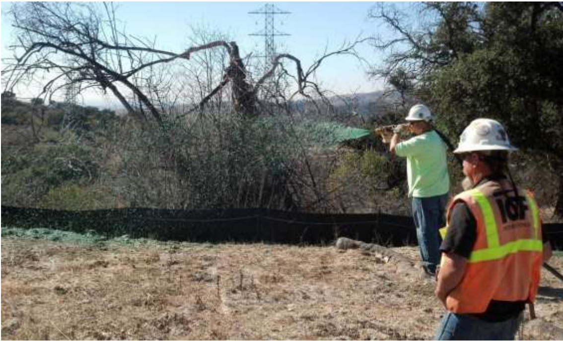
Figure 5: Wilson crew applying tackifier as a BMP to reduce erosion at M57-T4, Segment 8, Phase 1.
