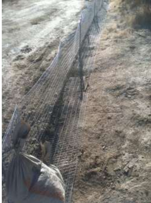
Figure 1: Segment 4 desert tortoise exclusionary fencing installed along the access road to Construct 2.
