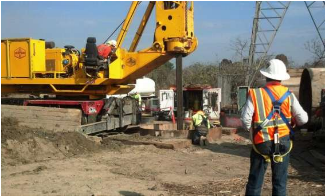
Figure 5: Tri-State drilling crew excavating a foundation hole at M41-T4, Segment 8, Phase 4, in Whittier Narrows Natural Area.
