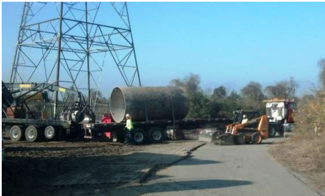
Figure 8: A street sweeper cleans the access road at M42-T1, Segment 8, Phase 4, in Whittier Narrows.
