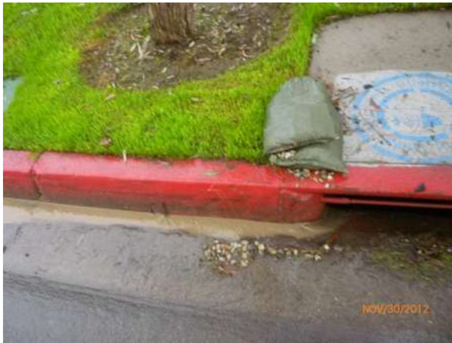
Figure 7: Sediment-laden water entering a municipal storm drain near the 605 yard entrance.
