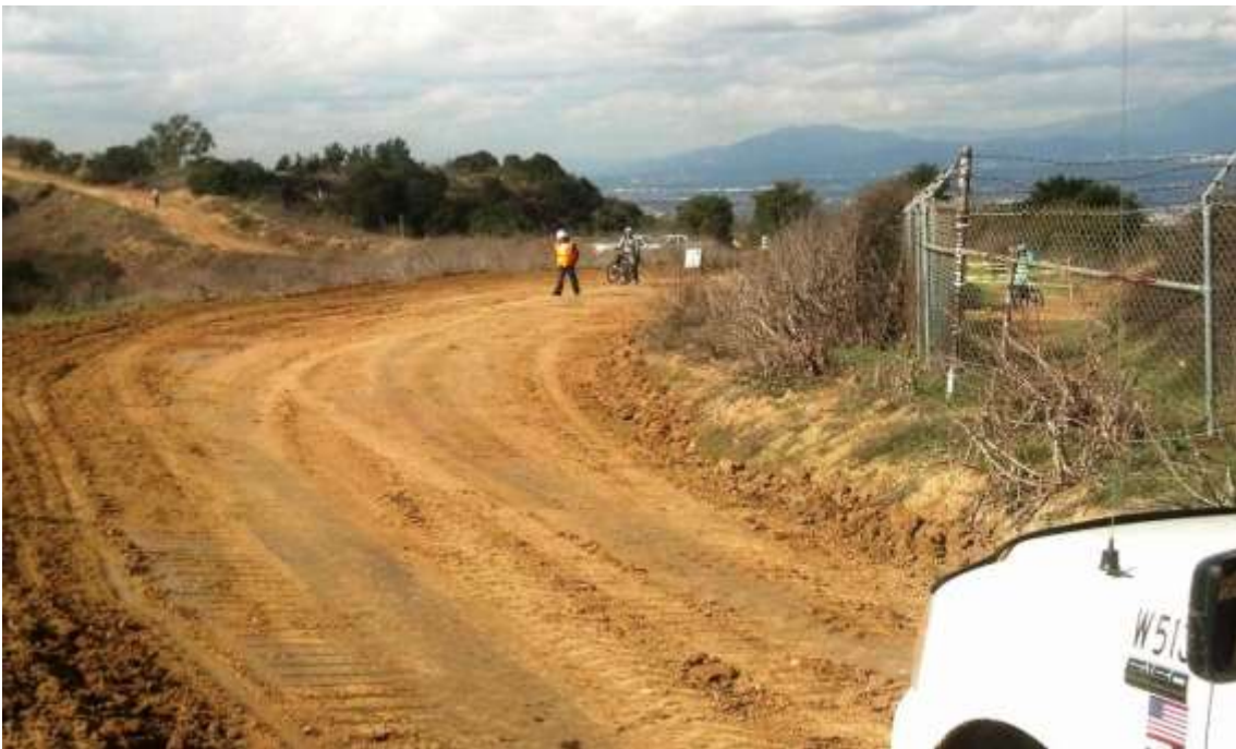
Figure 4: A worker escorts members of the public through the work site at M45-T4, Segment 8, Phase 4.
