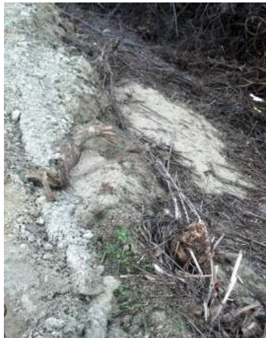
Figure 6: Sediment from a Baker tank that was emptied and exited the work area at M42-T1A in Whittier Narrows Natural Area, Segment 8, Phase 4.
