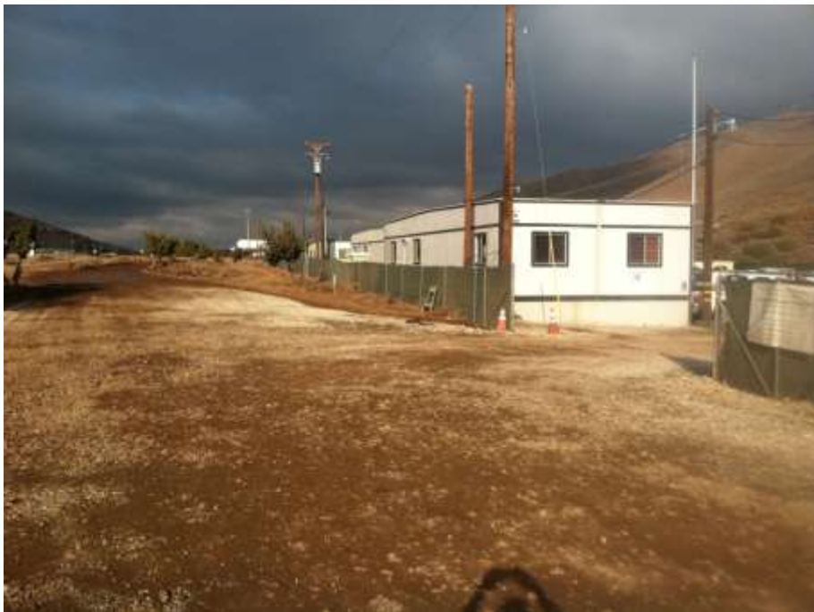
Figure 2: Stabilized construction area of Vincent Yard North that was noted to have been filled with soil prior to storm arrival on January 24, 2013.
