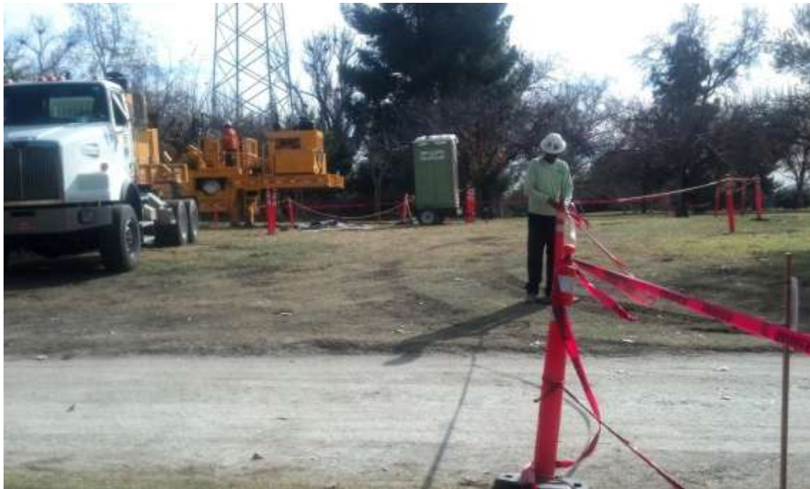
Figure 4: A worker directs the public around the wire pull area in Whittier Narrows Park between M38-T5 and M39-T4 per the related TEWS requirements.
