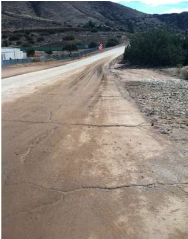
Figure 1: Track-out noted from Vincent South Yard.
