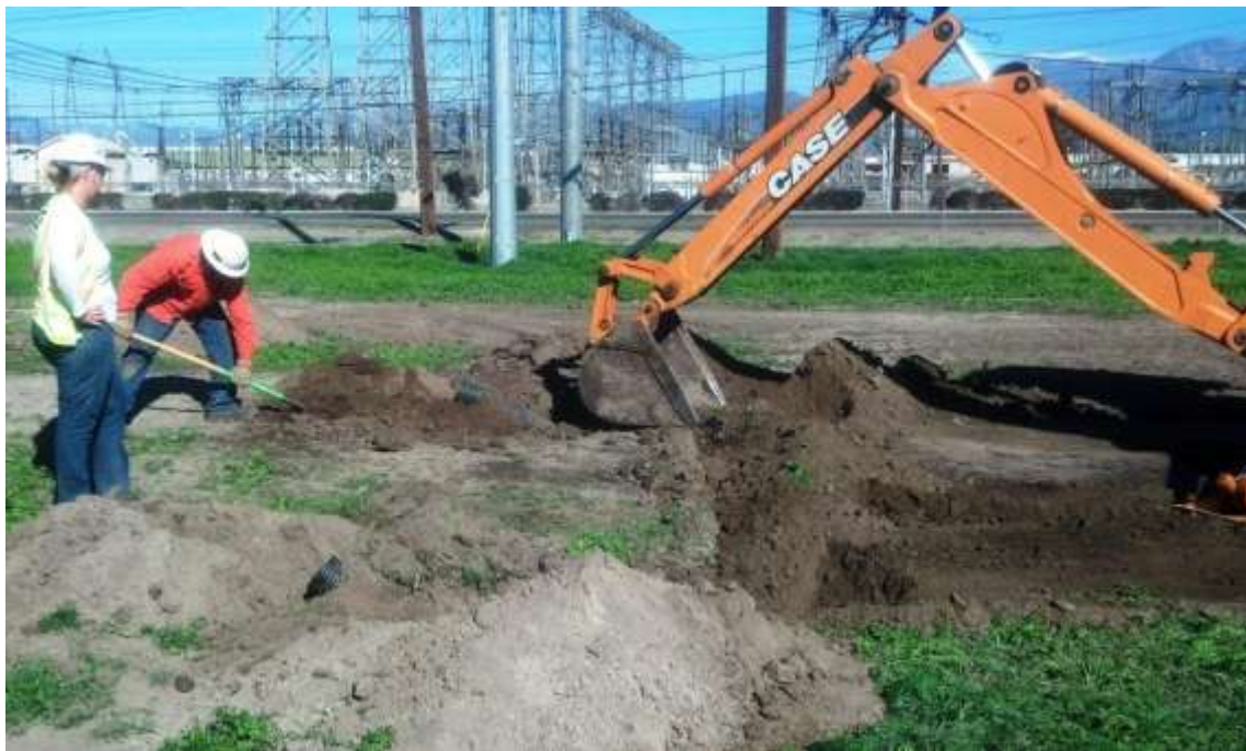
Figure 6: Workers and biologists install artificial burrowing owl burrows in Ayala Park near Tower M66-T6, Segment 8, Phase 3 in Chino, CA.
