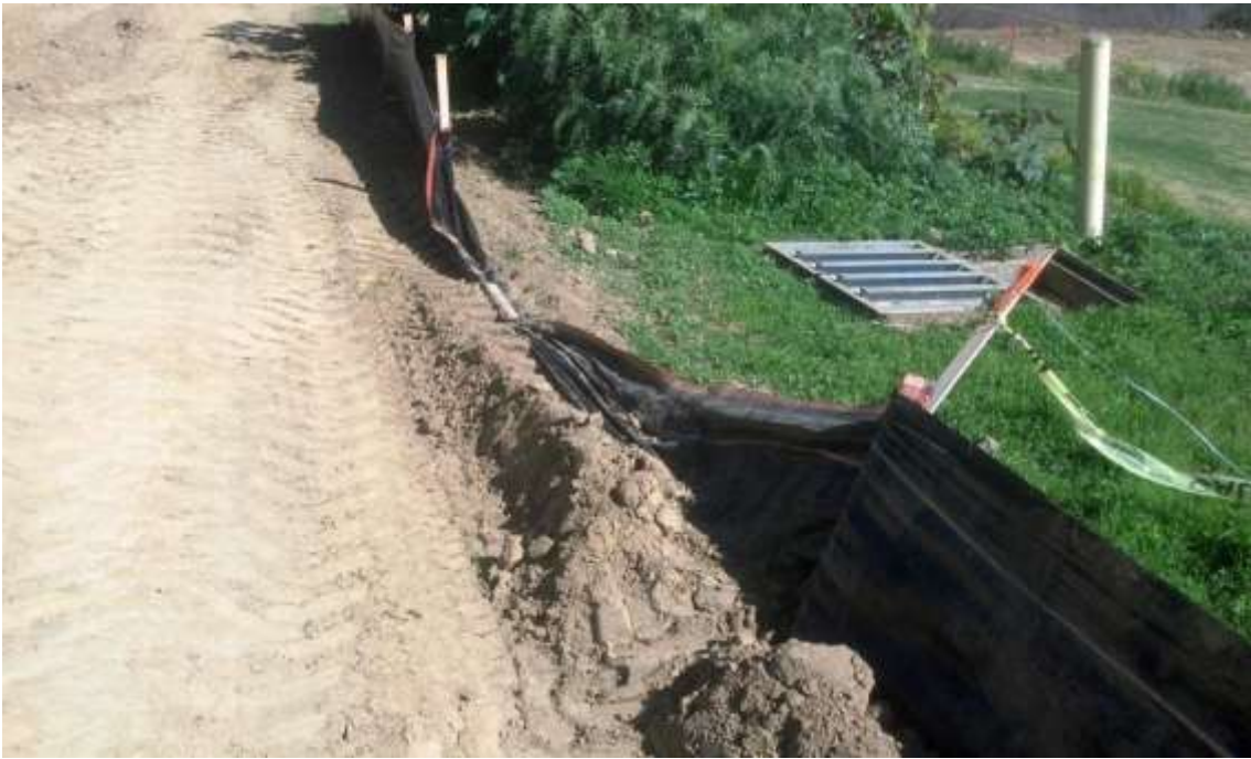
Figure 5: Silt fence knocked down at M44-T2.
