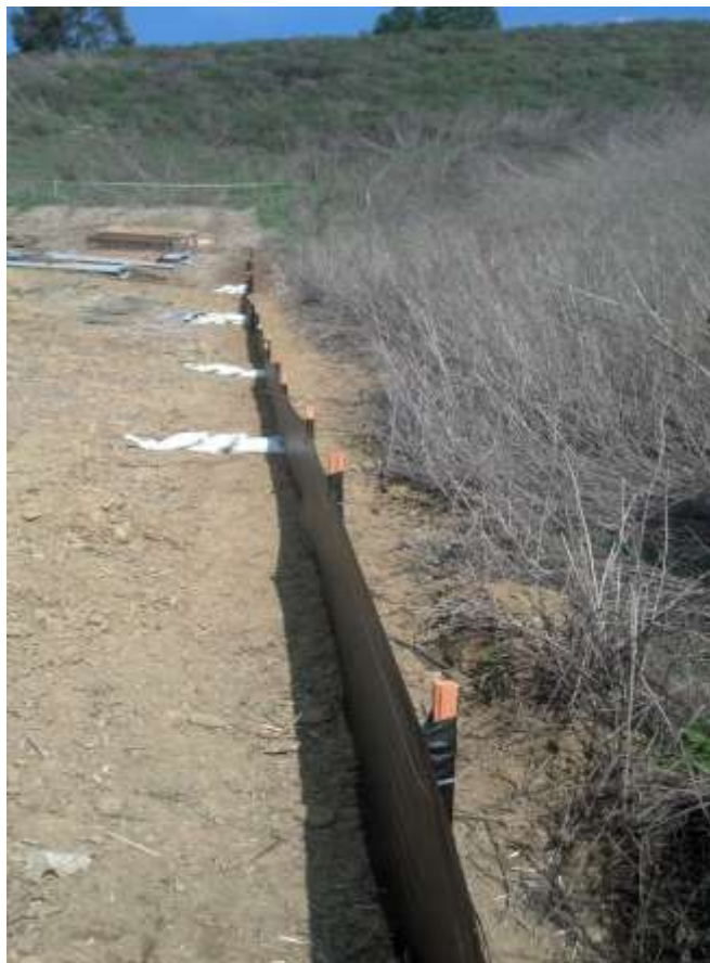
Figure 4: Silt fence and sandbags installed at the shoofly area in Rose Hills near M44-T2.
