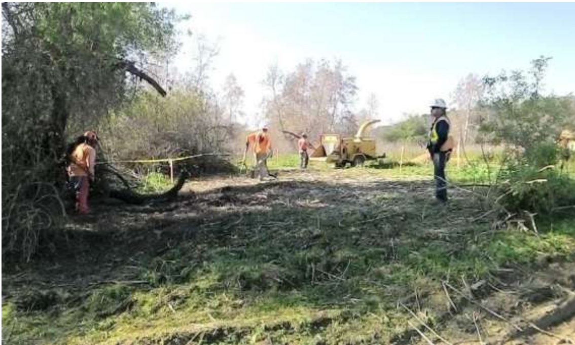
Figure 4: A Biological Monitor looks on as a crew removes vegetation near Tower M40-T5.
