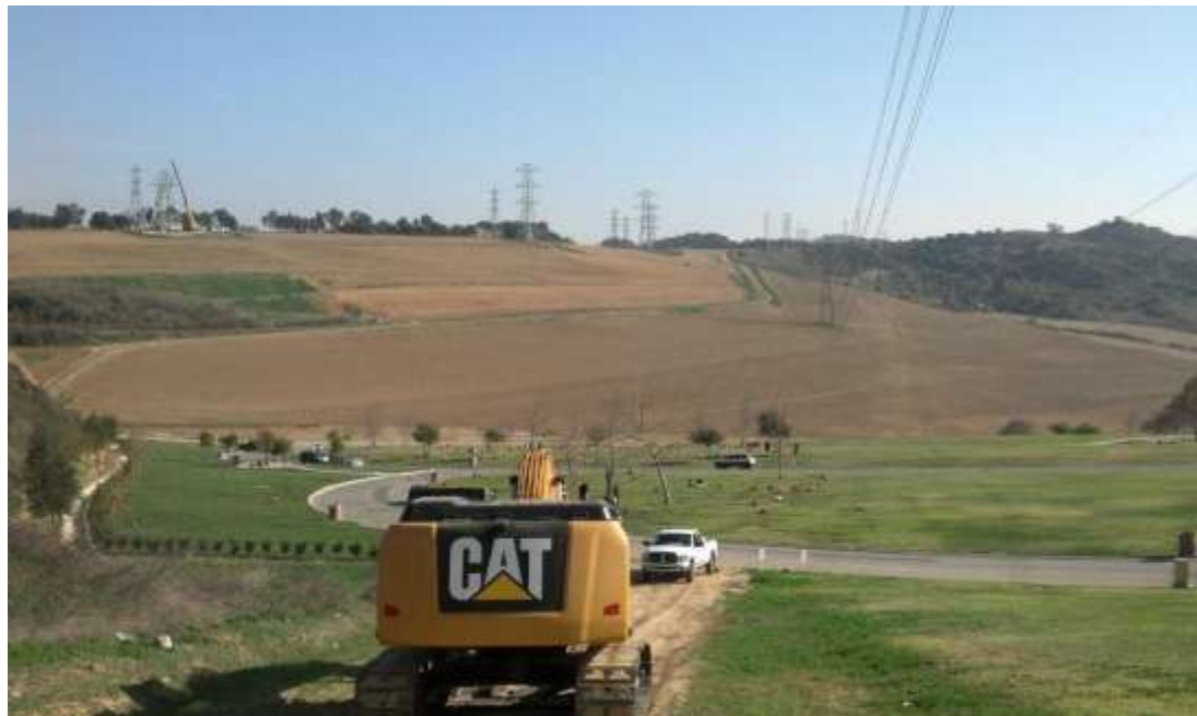
Figure 4: View south from Rose Hills shoofly with tower erection occurring at M45-T1 in the background, Segment 8, Phase 4.
