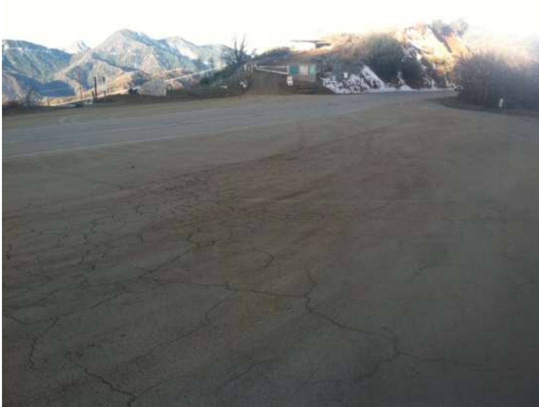
Figure 3: Visible trackout from Loop Road L prior to start of work.
