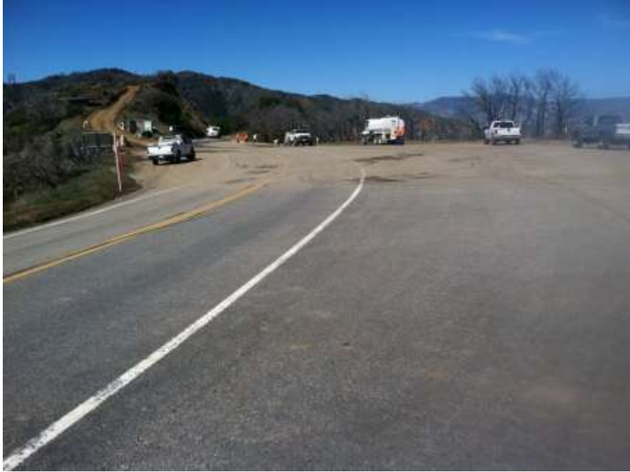
Figure 1: Trackout material from Loop Road L.
