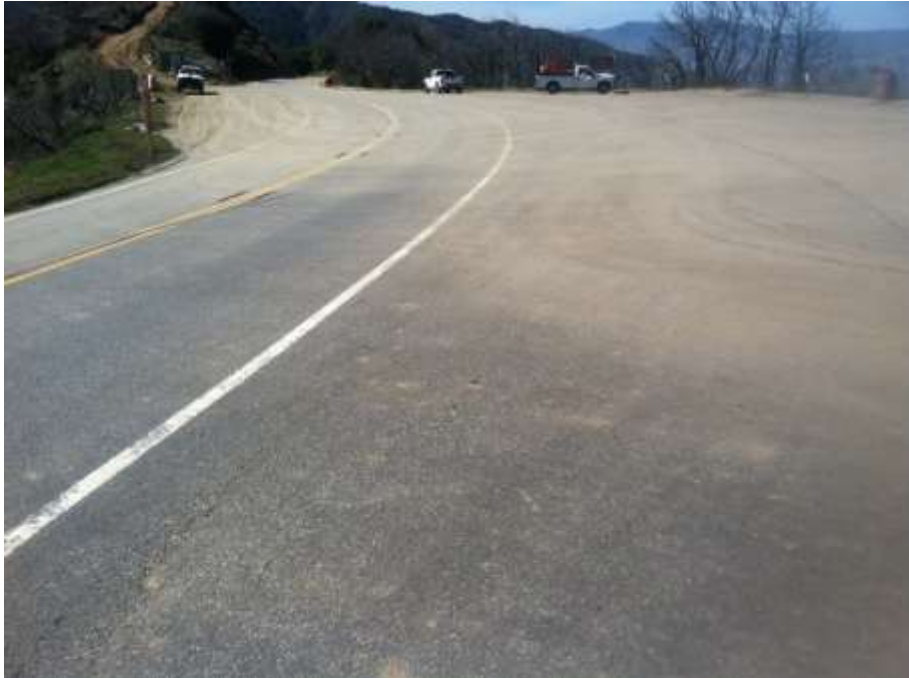
Figure 2: Trackout material from Loop Road L.
