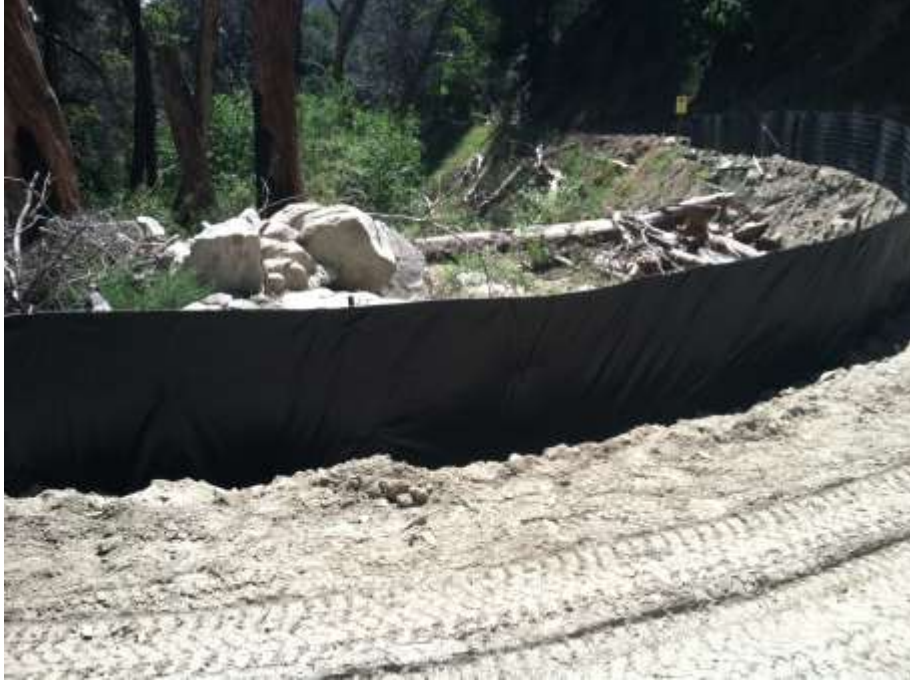
Figure 1: Silt fencing installed around drainage during road widening along Loop Road L, Segment 6C.
