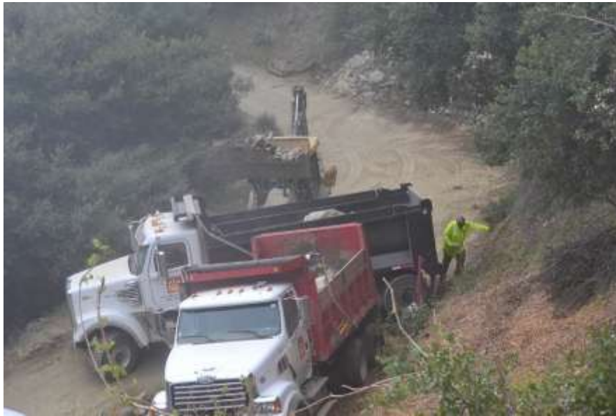
Figure 3: Rock removal along Loop Road L, trucks are removing the material from the USFS lands and trucking it to an offsite quarry.
