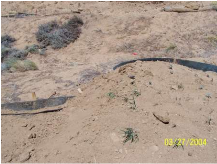
Figure 3: Segment 3B SWPPP failure at Construct 34.
