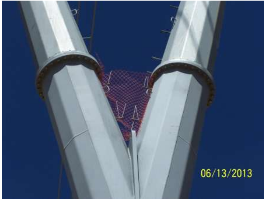
Figure 1: Netting within Structure 38 used to deter bird nesting during construction of Segment 3B is still present.
