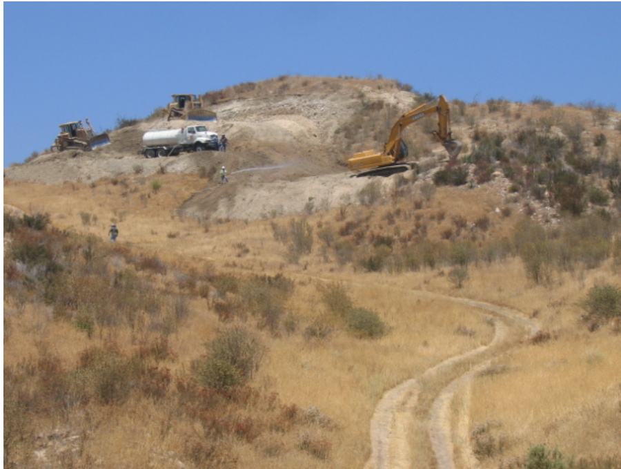
Figure 1: New road and crane pad construction at NC 26a, 26b, and 26c.
