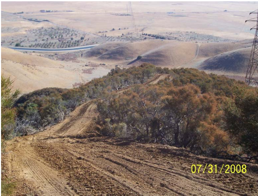
Figure 5: One Section 3 access road was improved in order for 12 kV crews to access a steep area.
