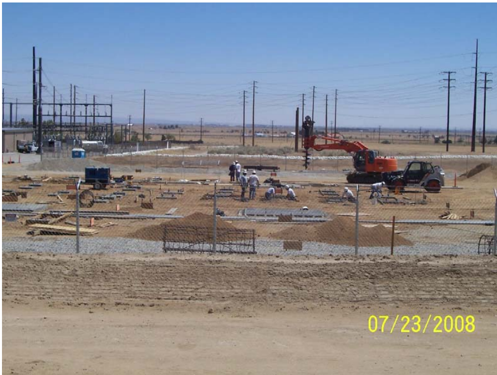
Figure 3: At the Antelope Substation, construction of the new components is taking place within the expansion area.
