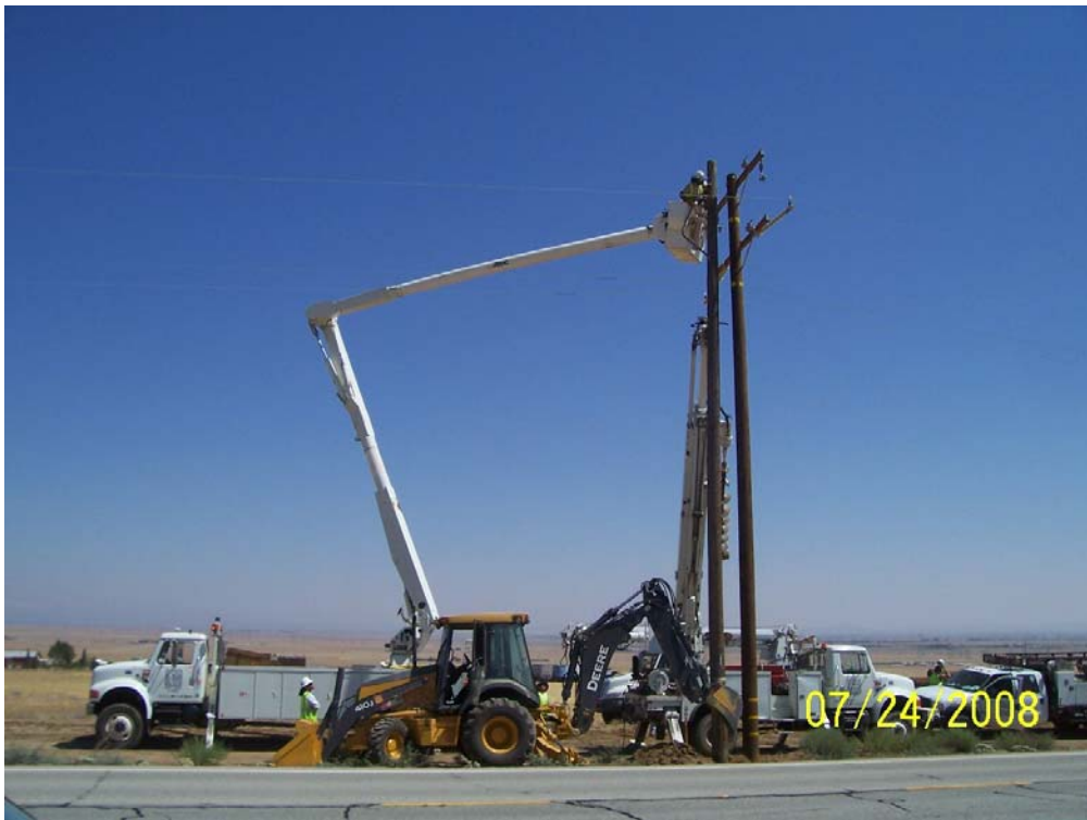
Figure 4: Pole setting for the 12 kV distribution line along Avenue K in Lancaster.
