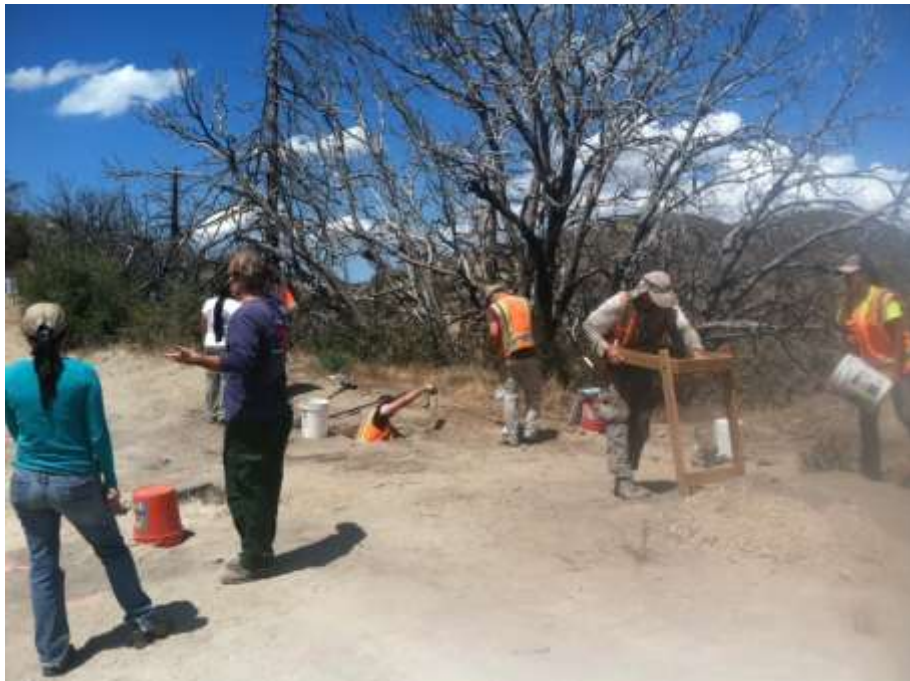
Figure 2: Cultural/archeological agency review with SCE throughout Segment 11C at site testing locations.
