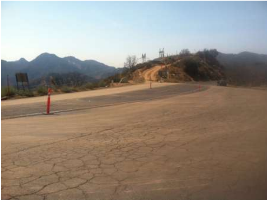
Figure 2: Trackout observed from Loop Road L along Angeles Crest Highway on Segment 6.
