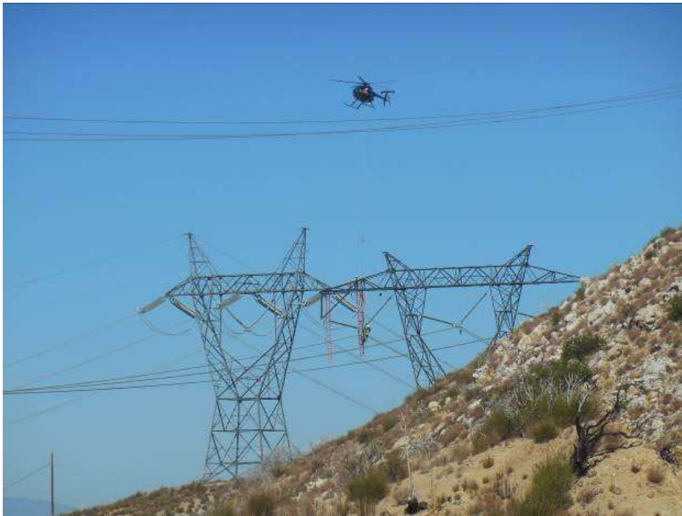
Figure 2: Helicopter transporting equipment during wire stringing activities between Constructs 22 and 28 along Segment 6.
