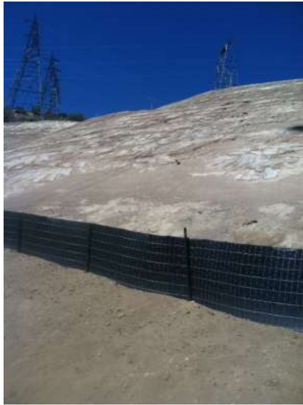
Figure 5: Construct 5 work area with no mid-slope BMPs as described in Segment 6A SWPPP.
