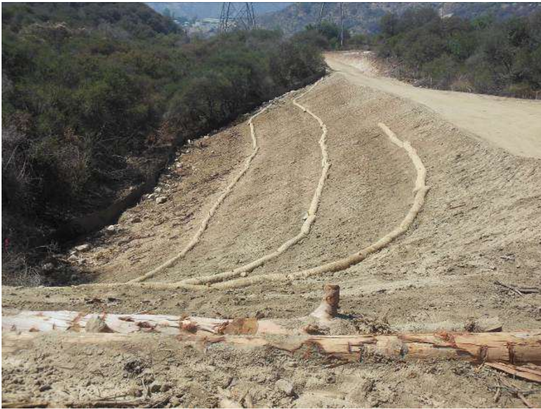
Figure 3: Newly installed fiber roll BMPs at the Chaney Trail Wire Stringing site along Segment 11B.
