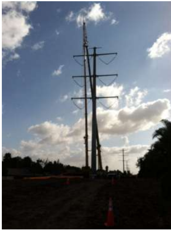
Figure 5: Demolition of previously installed TRTP structures in Chino Hills to prepare for the undergrounding project.
