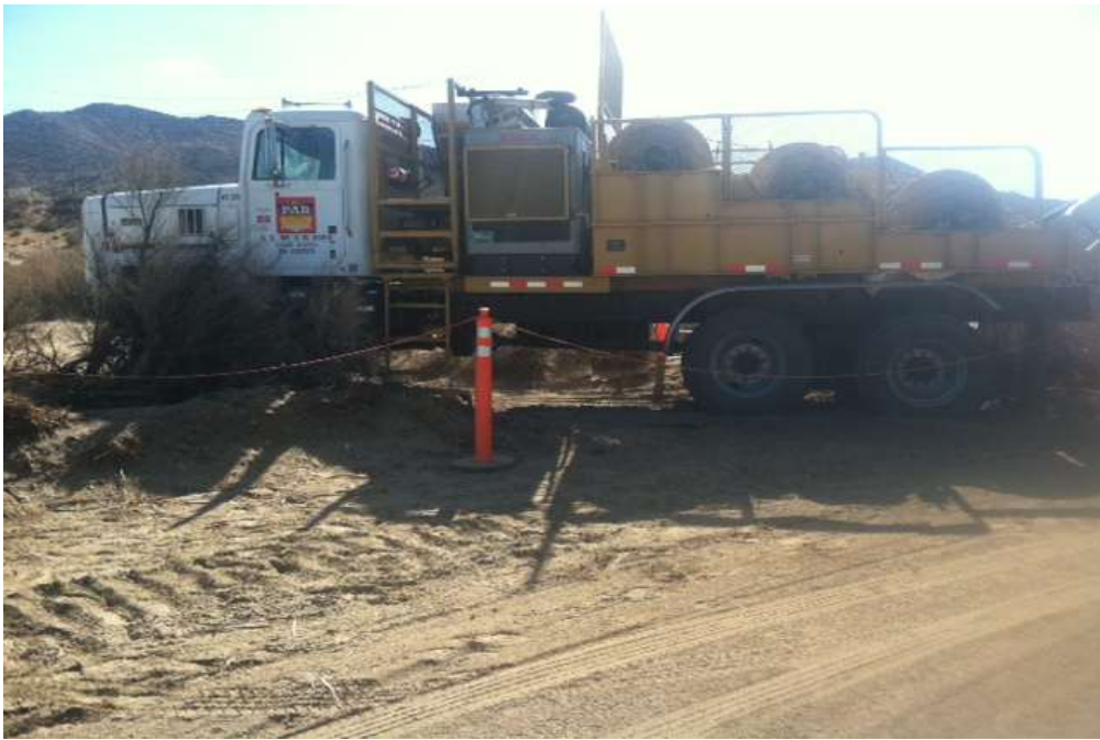
Figure 3: Wire equipment parked in unapproved work space near Construct 2 on Segment 6.
