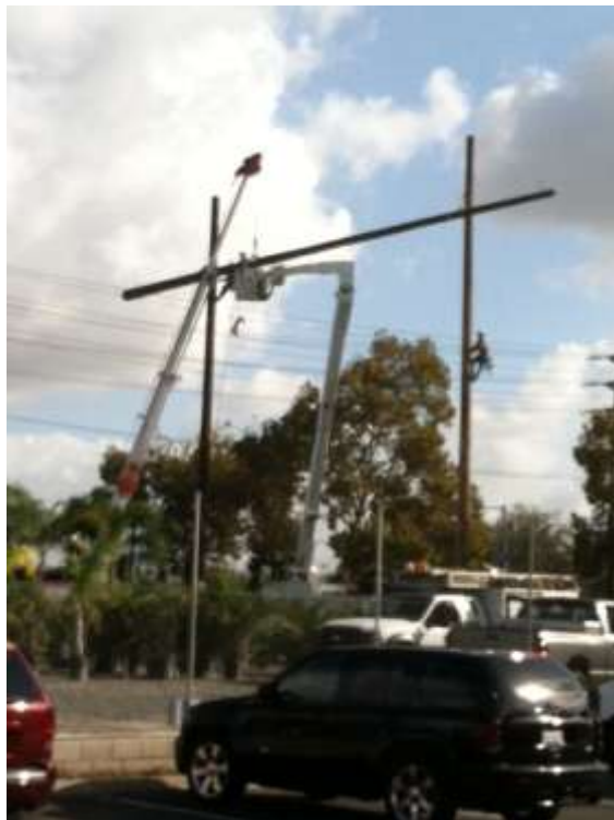
Figure 6: Removal of guard pole structures in place during wire removal in Segment 8 Phase 3 near Chino.
