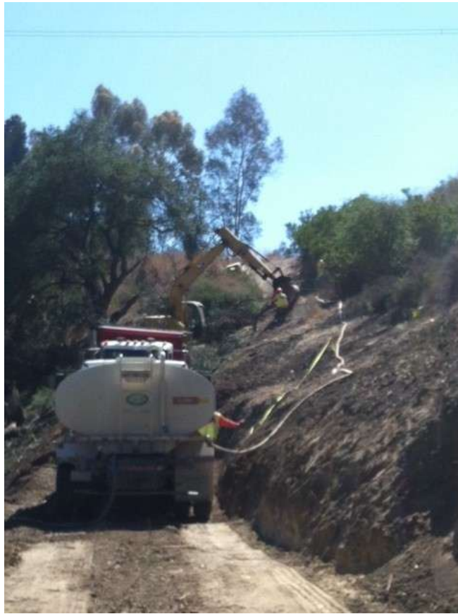
Figure 7: Vegetation clearing and grading of access road to Tower M49-T1 in Segment 8, Phase 4.
